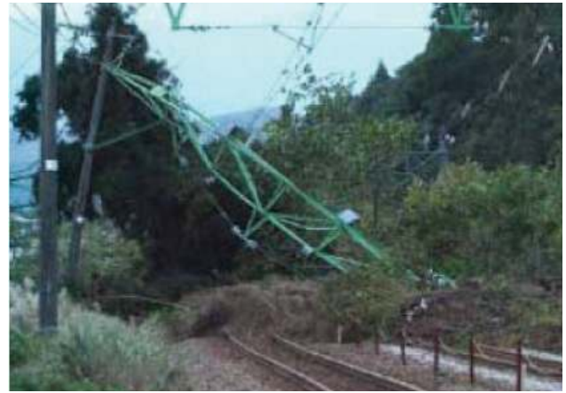
(b) overturn of poles on soil trackedbed
