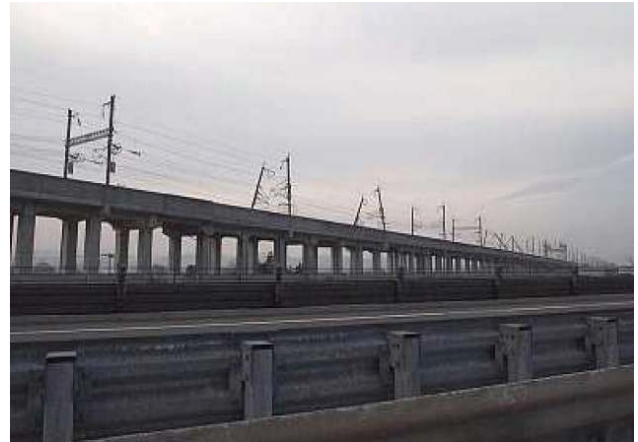
(a) overturn of poles on a bridge
