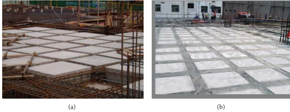
FIGURE 1: Construction procedures for a hollow-ribbed floor. (a) Locate prefabricated hollow box-like modules between the reinforcement grids. (b) Cast reinforced concrete beams between the box-like hollow modules.
