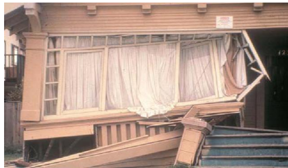
Figure 2-5: Failure of Cripple Wall in Loma Prieta Earthquake (Photo: C.Stover, U.S. Geological Survey)
