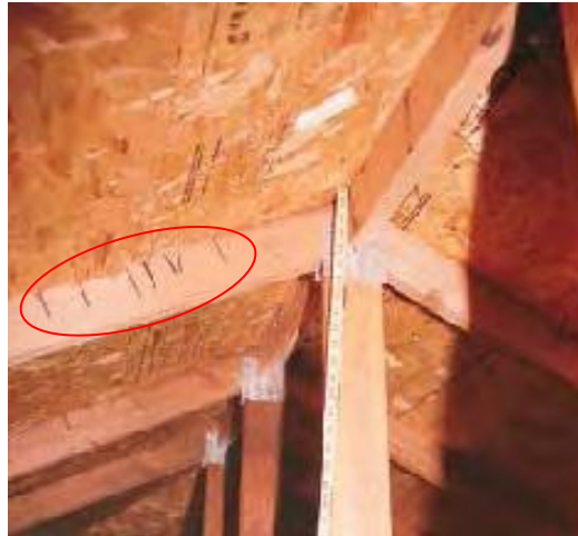
Figure 2-8: Nails Missing the Truss (Fowler, 1998)
