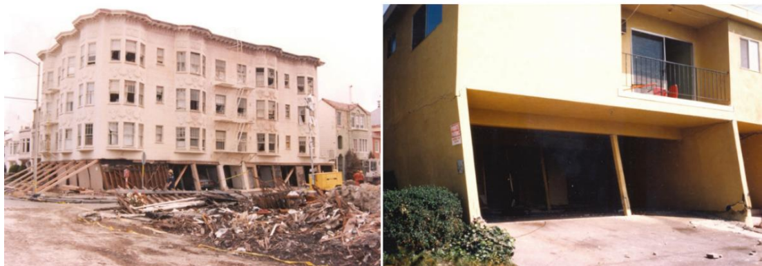
Figure 2-7: Failure in a Typical Wood Frame Construction Caused by Soft Story, in Loma Prieta Earthquake (Left) and Northridge Earthquake (right) (ATC, 2012)
