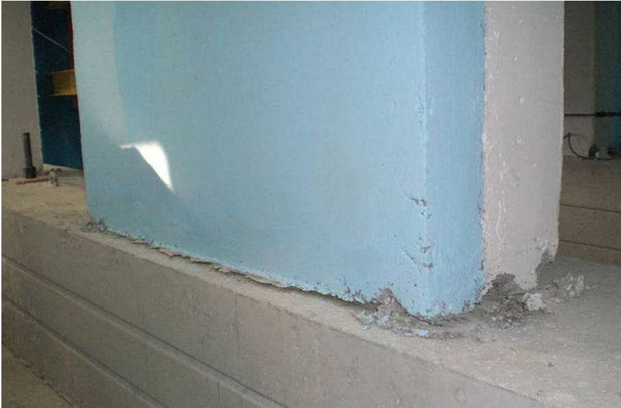
Figure 10. Concordant behaviour of the connecting column and the new shear wall.
