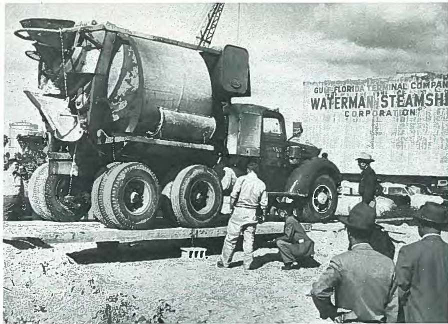
Fig. 24. Demonstration test by Cone Brothers Construction Co. in Tampa, Florida (1954) of 2-in. (51 mm) thick prestressed slab with 4-in. (102 mm) composite topping. The span was 30 ft (9.2 m) long.
