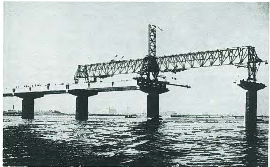
Fig. 29. The Champlain Bridge under construction: the largest application of prestressed concrete in Canada, and the most impressive from the viewpoint of low cost.
