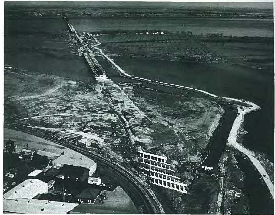
Fig. 28. An overview of the Champlain Bridge over the St. Lawrence and the Seaway at Montreal (built 1959-1962).
