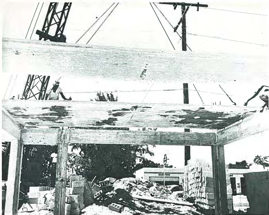
Fig. 9. Thin precast prestressed flat slabs were very popular in Florida in the mid-fifties. These particular slabs were 5 in. (127 mm) thick and 8 ft (2.44 m) wide with a span of about 20 ft (6.1 m), probably longer than would be allowed by today's codes.
