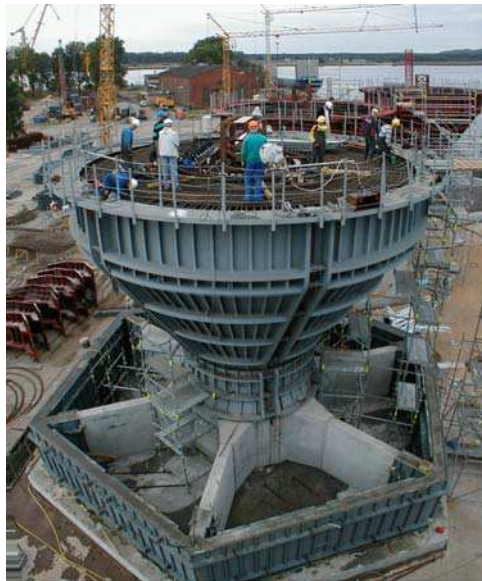
Fig. 7. Gravity Base Foundation being constructed for Nysted Offshore Wind Farm at Rødsand, Denmark. (Courtesy of Bob Bittner, Ben C. Gerwick, Inc.)
