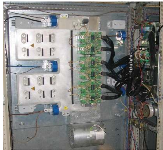
Fig. 5. 150 kVA IGBT-based back-to-back three-level diode-clamped inverter. The DC-Link voltage is 800V.
