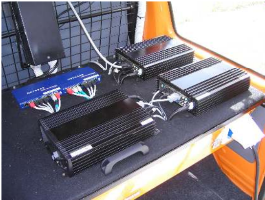
Fig. 5. The 3 onboard PCs installed into the booth of the first test vehicle.
