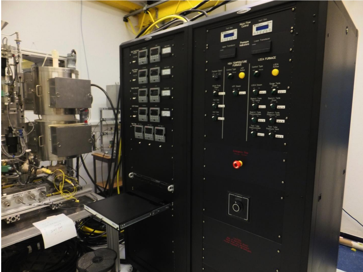
Figure 25 BDBA in-cell module located at hot cell facility
