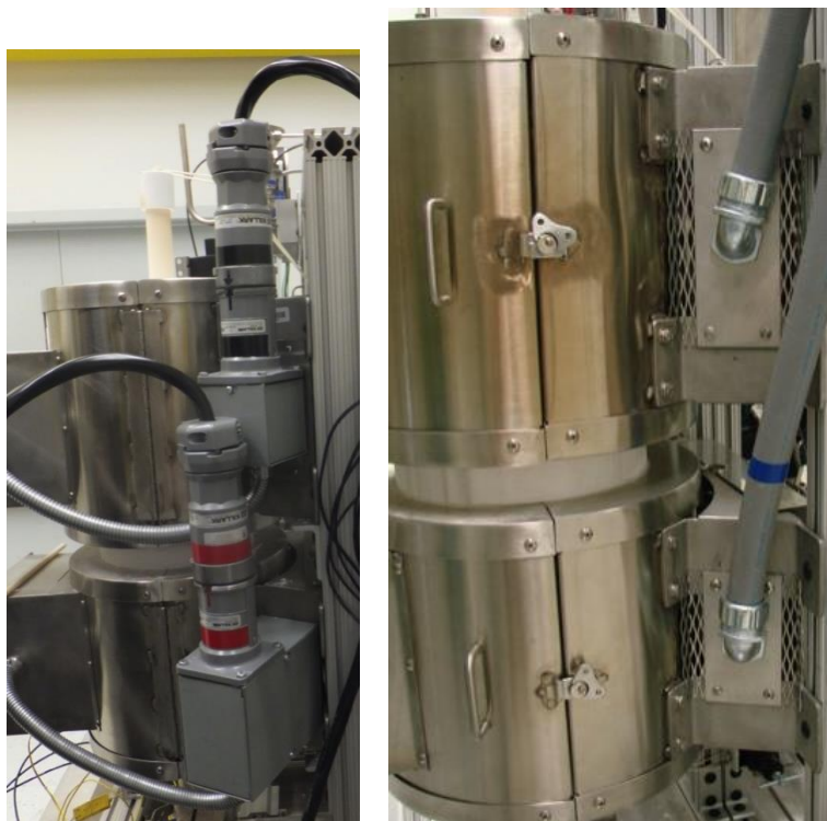
Figure 27 Power connections for the high temperature furnaces on the out-of-cell module (left) and in-cell module (right).
