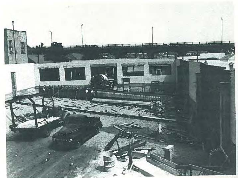
Fig. 22. Post-tensioned beams were cast on site at the Star Bakery because of the limitations of existing transportation equipment.
