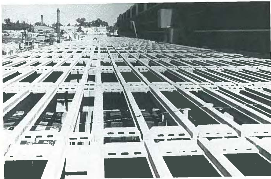
Fig. 13. Prestressed block joist and filler construction on 100,000 sq ft (9290 m 2 ) warehouse for Crosley Corporation. Joists are made continuous over 18 x 24-in. (457 x 610 mm) prestressed block beams by reinforcing steel in the topping slab.
