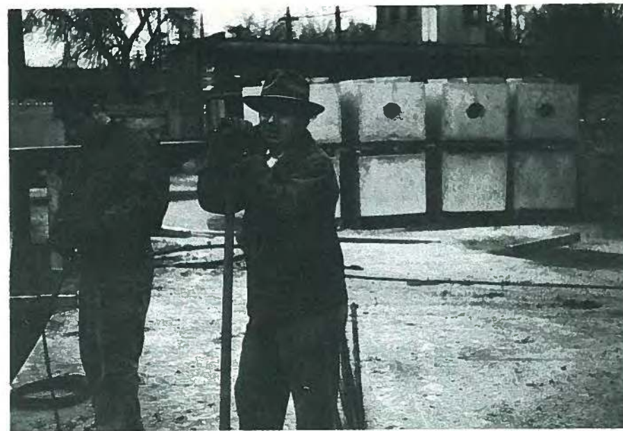
Fig. 5. Jack Perlmutter (right) and Michael Altenberg were among many men who worked day and night on Prestressed Concrete of Colorado's first pretensioning bed. The original 50-ft (15.2 m) bed was the beginning of the remarkable growth of prestressed concrete fabrication in Colorado.
