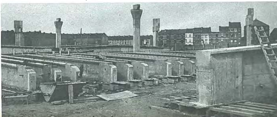
Fig. 33. Construction site of prestressed warehouse in Ghent, Belgium. The beams, cast on location, are ready to be hoisted into position.
