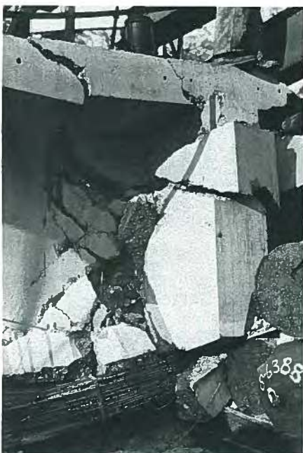
Fig. 12. Closeup of fracture zone of Walnut Lane test girder. Failure was in the top flange to right of the stiffener.
