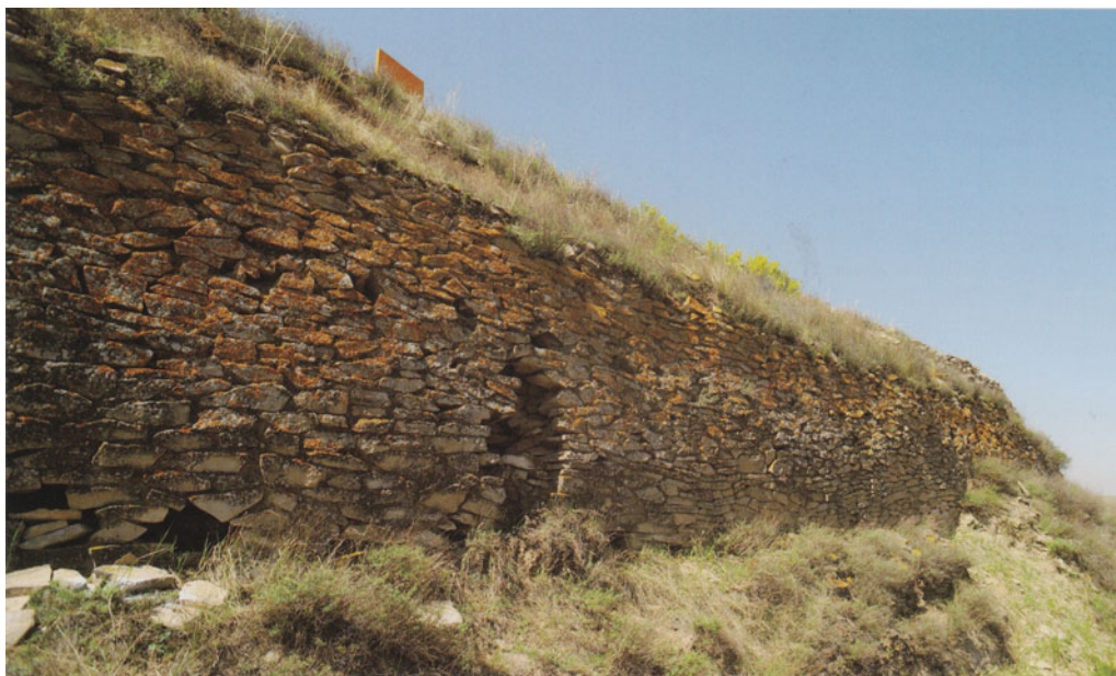
Figure 2. One of the major retaining walls at Shimao, after Faxian Shimao gucheng, p. 37 (upper figure).
