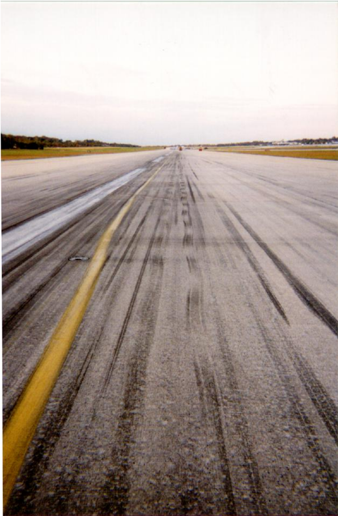
Fig. 6.1: Tyre marks on the runway (1).
