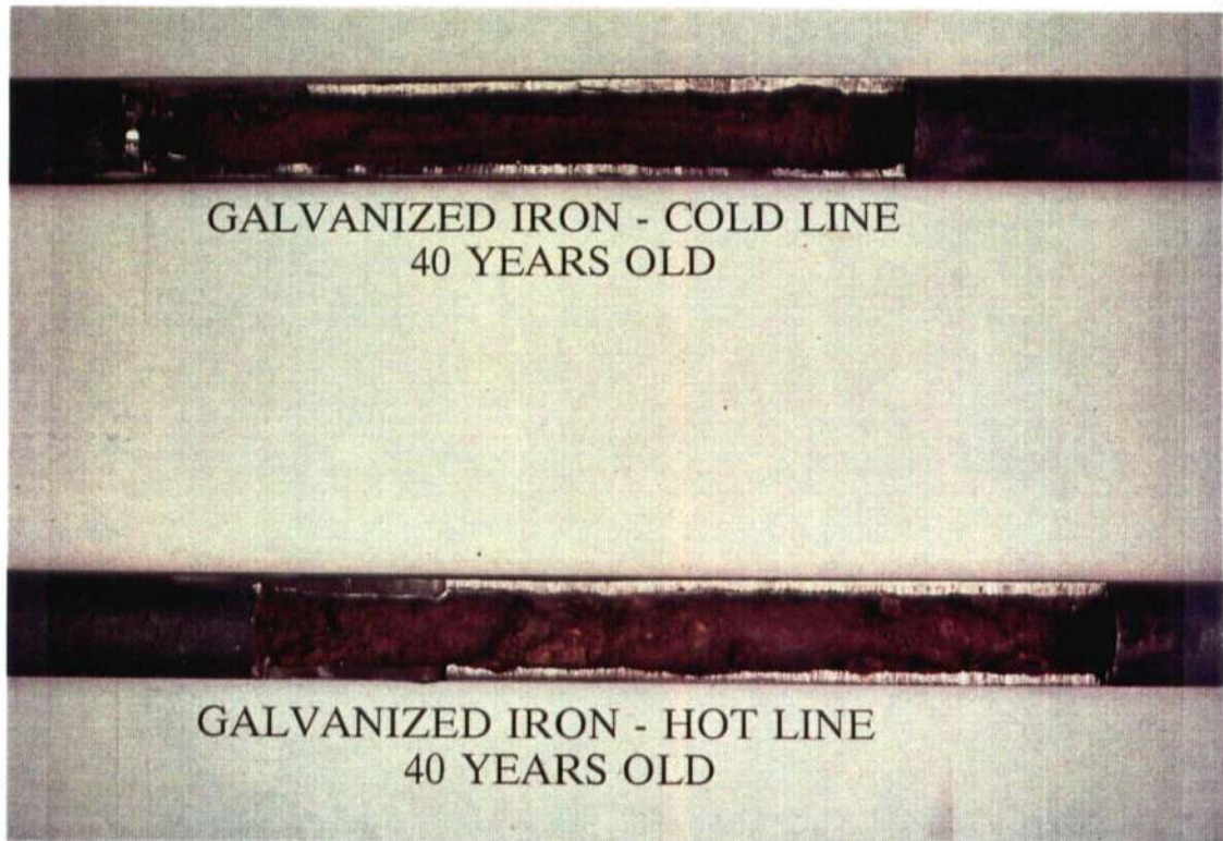
Figure 2-5. Tuberculation Inside Corroded Galvanized Iron Pipe
