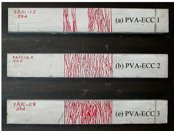
Fig. 12 Beam bottom surface shown increasingly saturated microcracks after bending test for PVA-ECC 1-3 (Microcracks are magnified with thick pen for the constant moment span length only).
