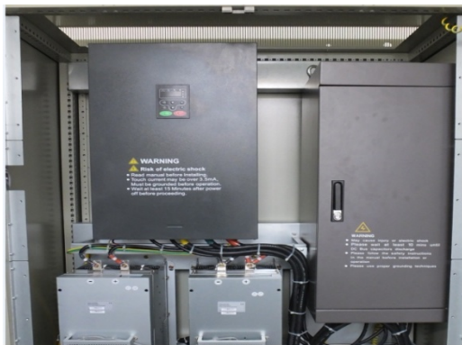
Figure 17. Picture of electric multi-drives equipment.
