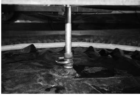
Figure 6: The membrane placed on the soil surface and sealed around the pile by hose clips and sealed against the side of the tank by a fire hose.
