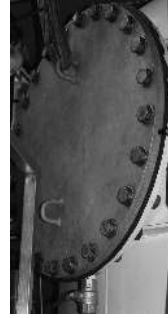
Figure 7: The openings in the tank hermetically sealed.
