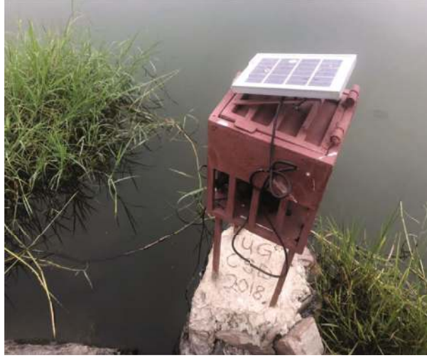
FIGURE 8: Externally mounted solar panel for energy harvesting in freshwater.
