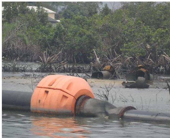
Plate 7. Picture showing damaged riparian vegetation Source: Authors' field survey, 2016
