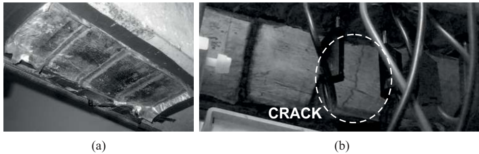
Figure 12: Vertical pattern ‘non-stacked’ sensor sheet used for the large-scale test: (a) deployed on the beam; and (b) a crack formed under a patch.
