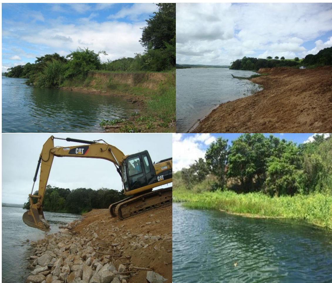
Figure 10. Lower São Francisco Riverbank recovery, Northeastern Brazil, through soil bioengineering technique called Vegetated riprap, from 2010 to 2018.
