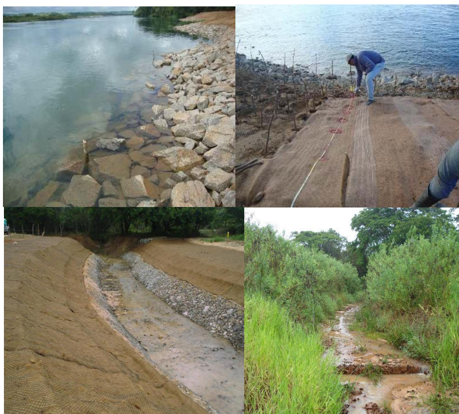
Figure 8. Use of geotextiles, with riprap and gabion as toe protection, on the banks of the São Francisco and Paramopama Rivers.
