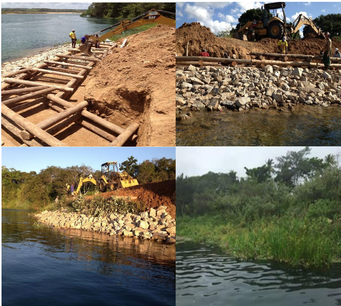
Figure 11. Lower São Francisco Riverbank recovery, Northeastern Brazil, through soil bioengineering techniques called Crib-wall, from 2013 to 2018.
