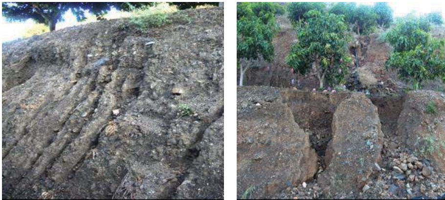
Figure 7. Rills and gullies in the taluses of orchard terraces.
