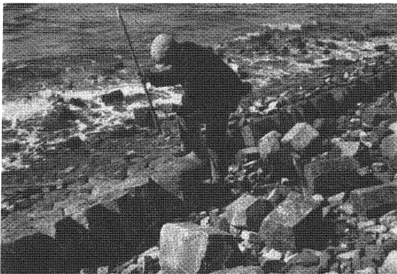
Figure 5.2 Construction of a block revetment on the Afsluitdijk, near Kornwerderzand (1927), © municipality of Wieringen
