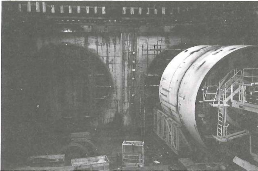
Figure 7.1 Tunnel boring machine installed for the start of the second Heinenoord tunnel
