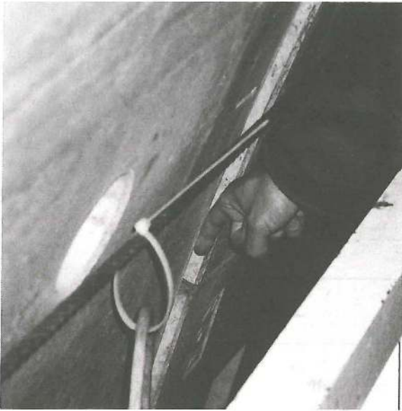
Figure 7.33 Differential displacement as observed at the Second Heineoord tunnel
