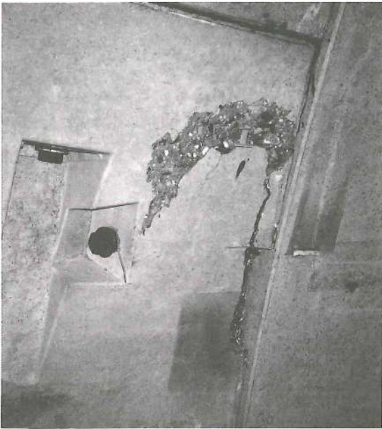
Figure 7.29 Damage to the tunnel lining; i.e. damage near the dowel and notch system
