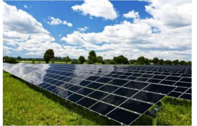
Fig. 2. Shaded solar array.
