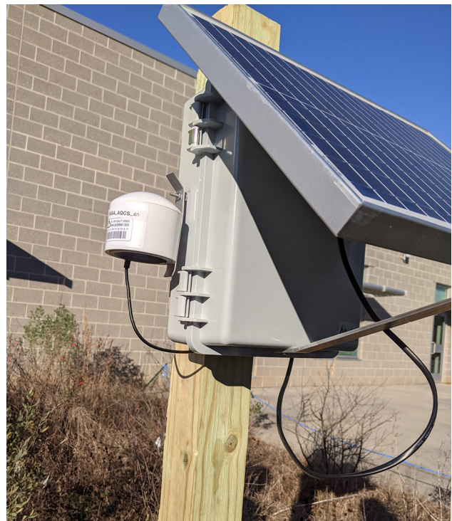
Figure 1. Solar station design used in RTI’s initial testing and deployment with the panel mounted to the waterproof box (prototype design)
