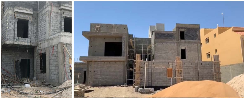
Figure 1. Concrete frame construction with block in-fill and example of villa-style housing development in Saudi Arabia.
