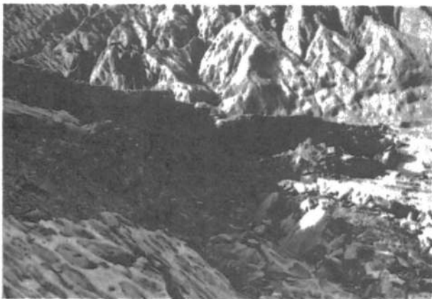
Fig. 11 Photograph of the slide on the upstream slope of Kashi earth dam at 0+250
