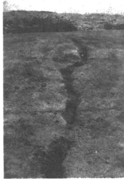
Fig. 2 Photograph of Changmaidi dam, transverse cracks on the dam.
