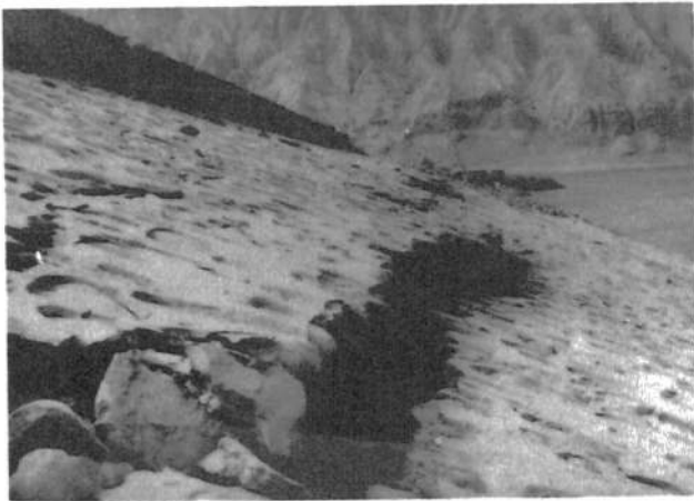
Fig. 8 Photograph of longitudinal cracks on the upstream slope of Kashi earth dam
