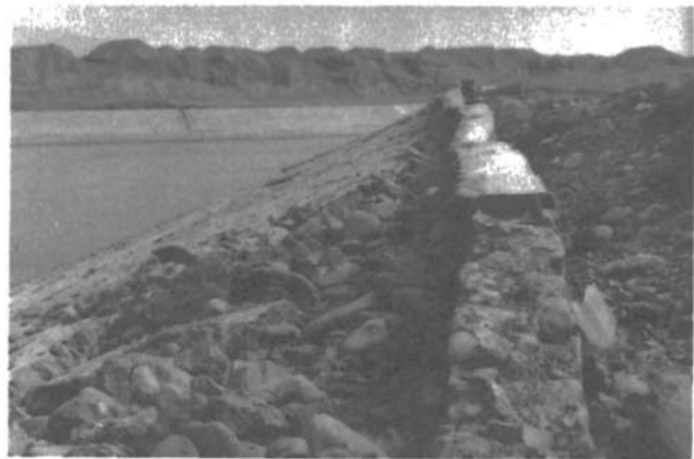
Fig. 12 Photograph of the failure of Parapet Wall on the crest of Kashi earth dam
