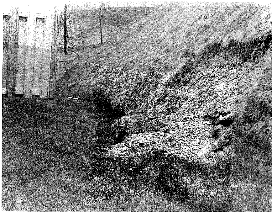
FIG. 8. Bulge at toe of slope behind row house 227 at 241 Le Coteau.
