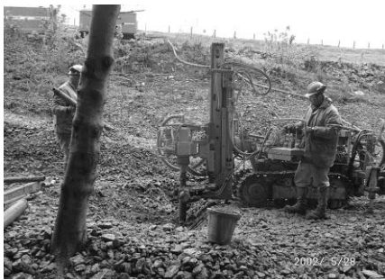
Figure 4. Mini track-mounted drilling rig operating on embankment slope. Note distorted tree trunk in foreground leaning down slope.
