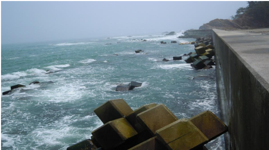
Figure 2. Failed X-Block Armour Units at Hikado Port
