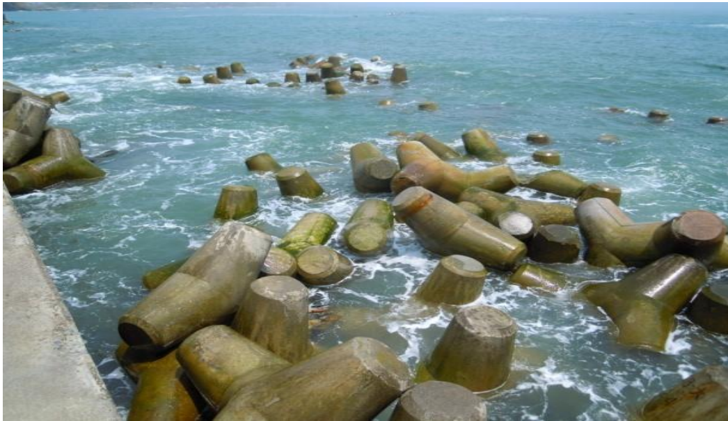
Figure 1. Damaged Sea-Block Armour Units at Ooya Port
