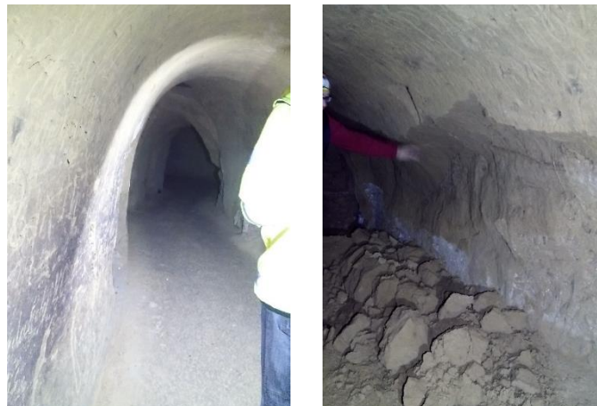
Fig. 4: The state of the Čachtice underground and a dangerous intervention in the statics.
