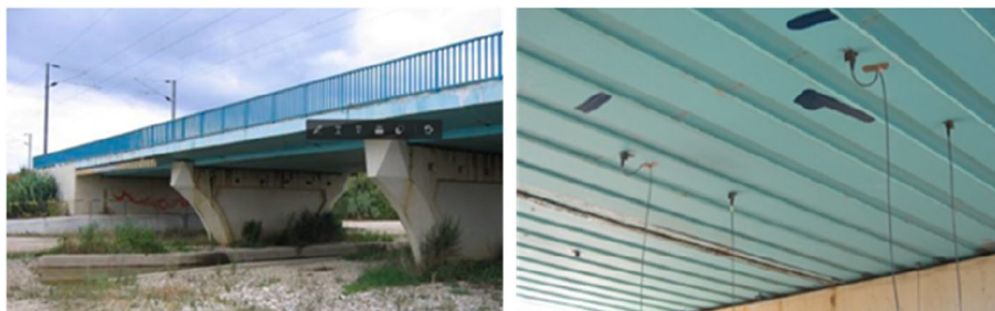
Fig. 27 The bridge dynamic weighing system
