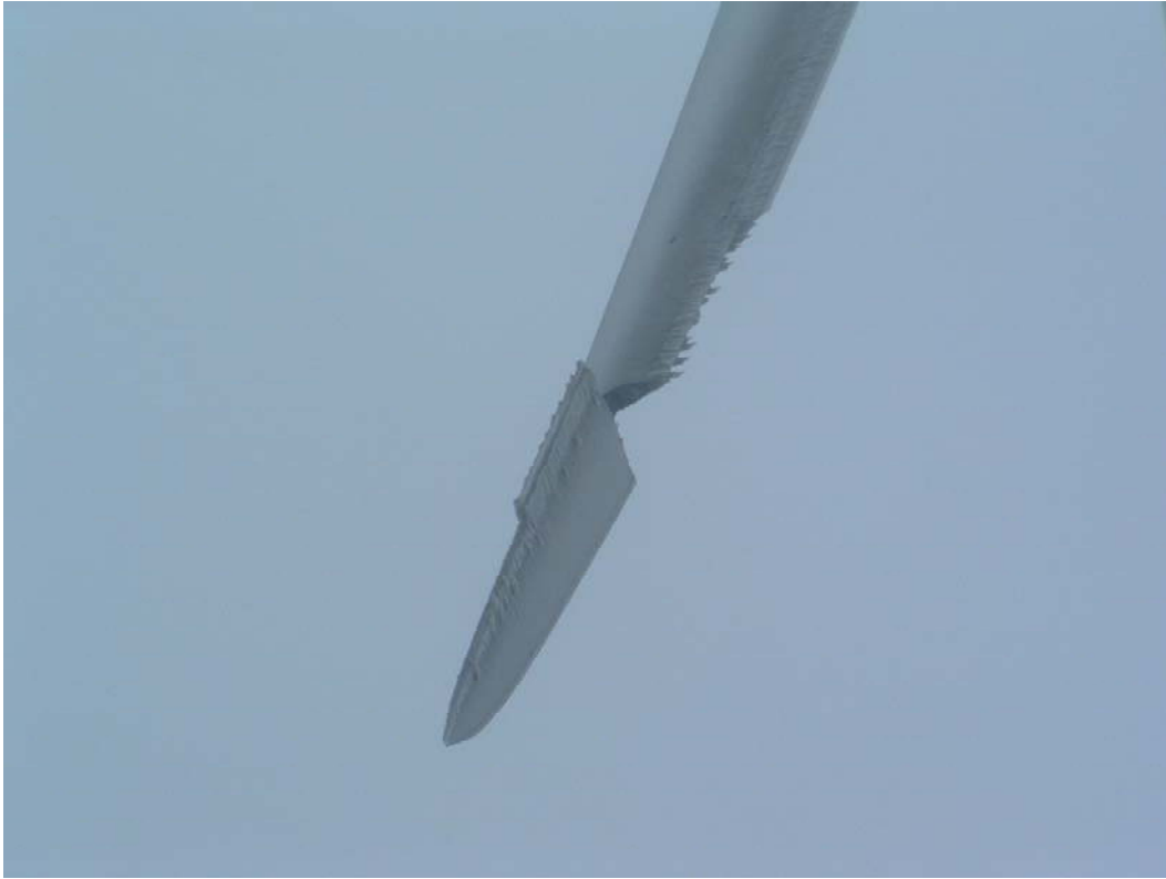
Figure 18. Ice build-up on a wind turbine blade during winter of 2002/2003.
