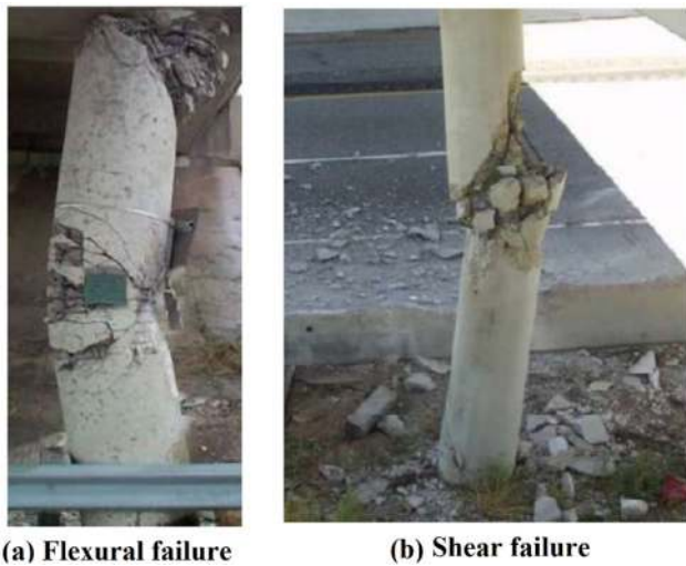
Fig. 10 Typical failures occurred in bridge columns at the mid-height under vehicle collisions [78]
