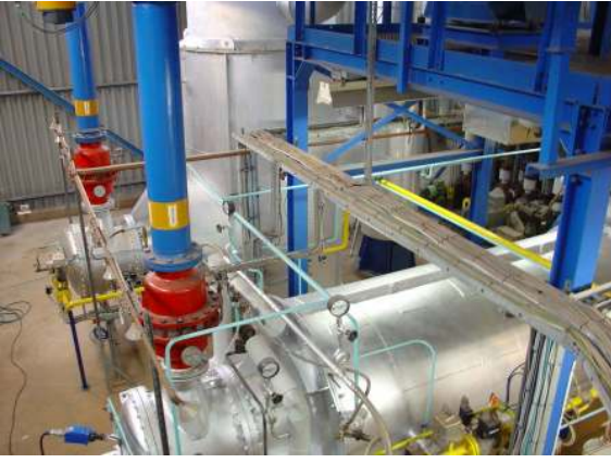
Fig. 1. A view of the incinerator hall, showing the metallic environment as seen from the balcony.
