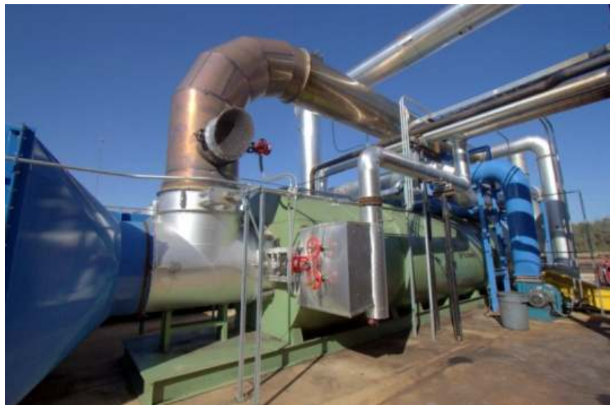
Figure 7.8 One of the hot oil systems at the NBE plant
