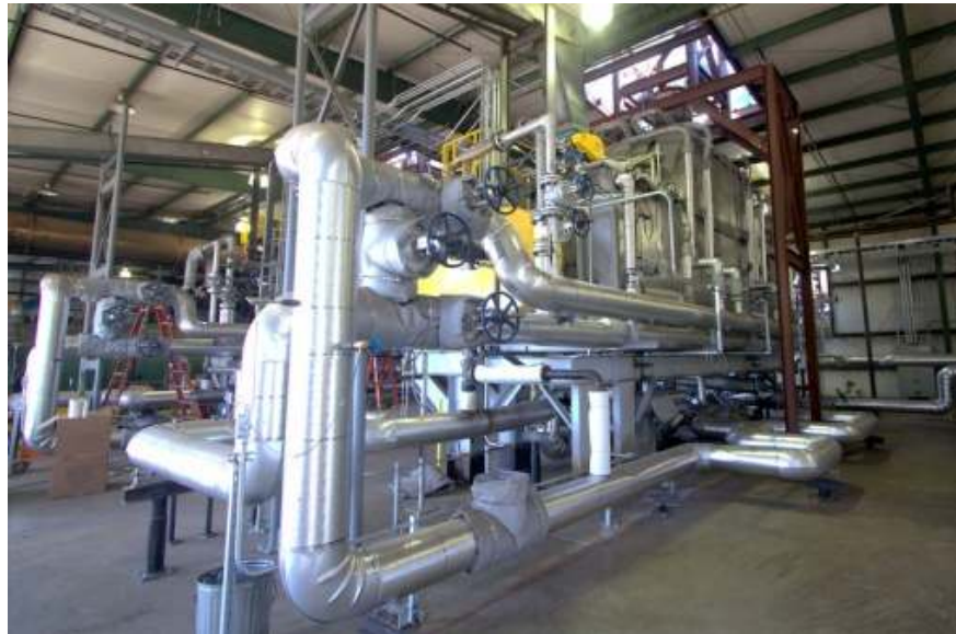
Figure 7.7 The NBE torrefaction Reactor
