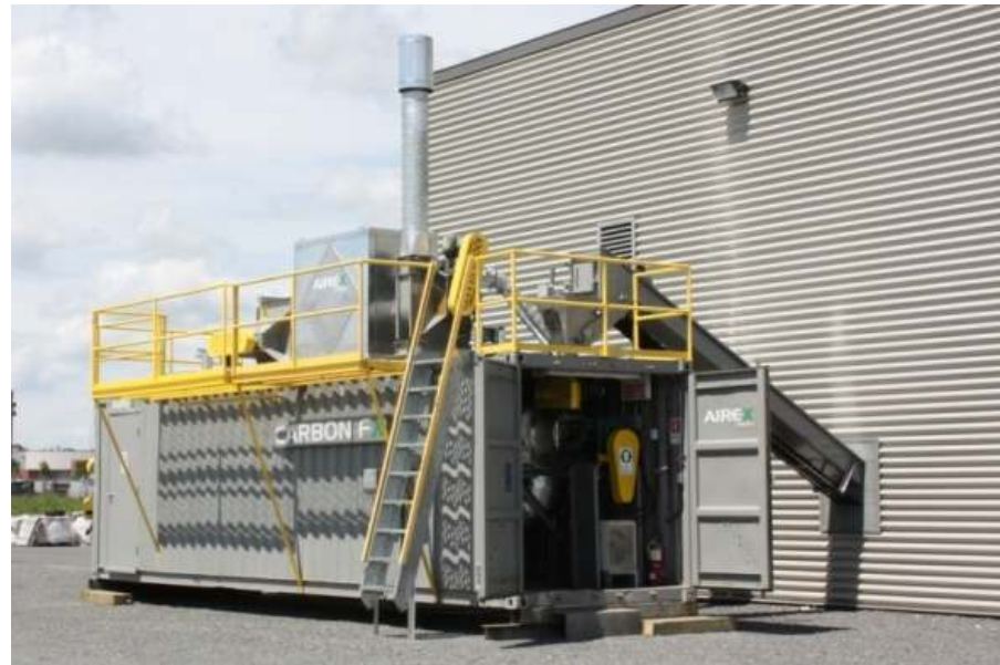
Figure 7.4 Cyclonic reactor and combustor of the Airex installation.
