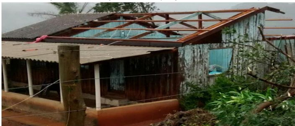
Figure-3. Photo of damage caused at home by alleged Tornado in Rosario do Ivaí [3].
