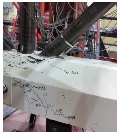
(c) Concrete crushing at bottom chord
