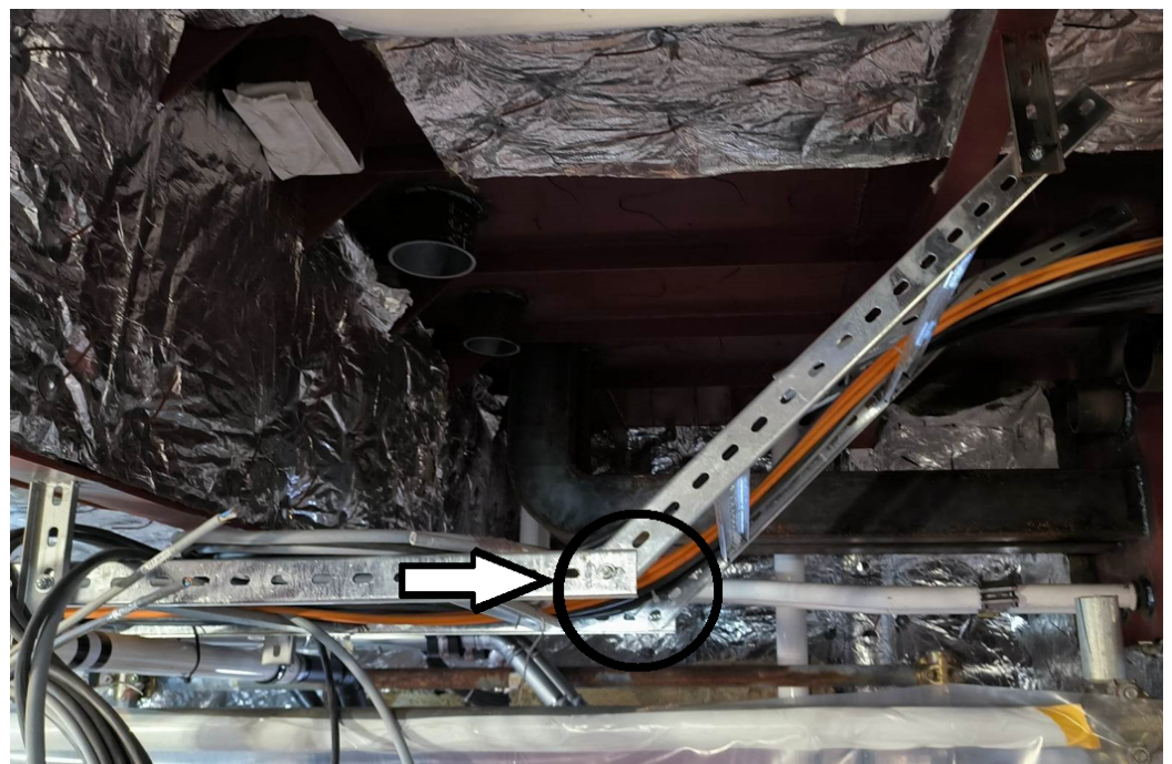
Figure 3. Cable tray with indicated bolted joint.
