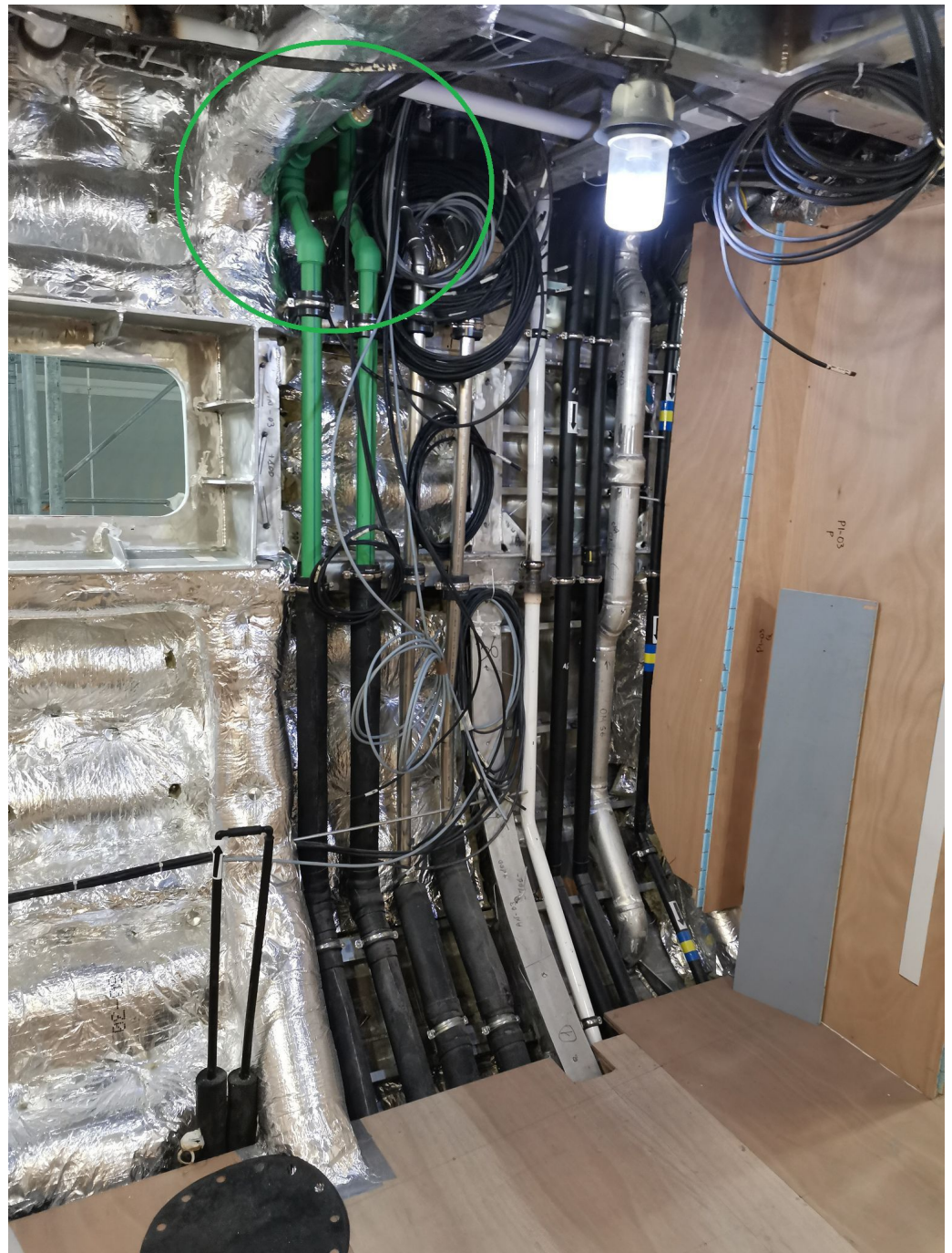
Figure 6. Example of installed redundant elbows on the ship.
