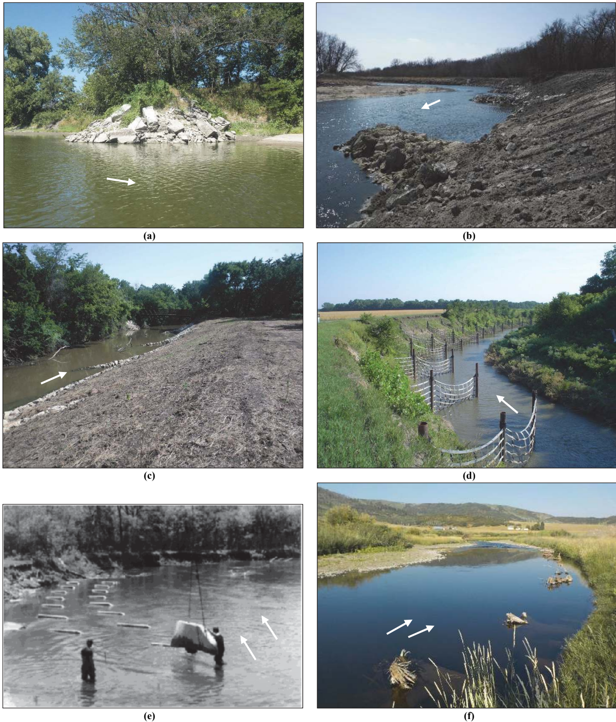
Figure 1. Examples of streambank stabilization techniques (white arrows indicate flow direction): (a) impermeable spur on Kansas River, Kansas, (b) bendway weirs, toe rock, and streambank shaping on Big Blue River, Kansas, (c) rock vanes, toe rock, and streambank shaping on Cowskin Creek, Kansas, (d) permeable spurs on Solomon River, Kansas (photo courtesy of Wildhorse Riverworks, Inc.), (e) concrete submerged vanes (photo from Iowa DNR, 2006), and (f) woody revetment/toe wood, bankfull bench, and planted vegetation on Yampa River, Colorado.
