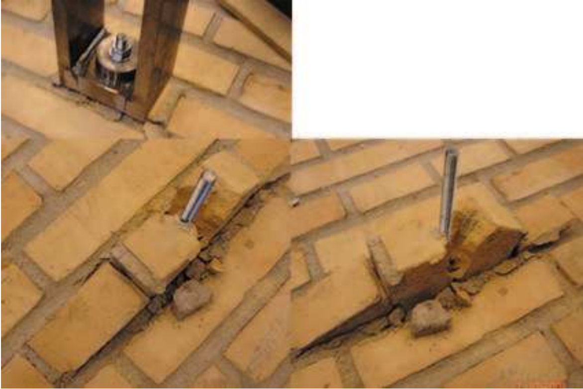
Figure A.43: The failure mode observed
