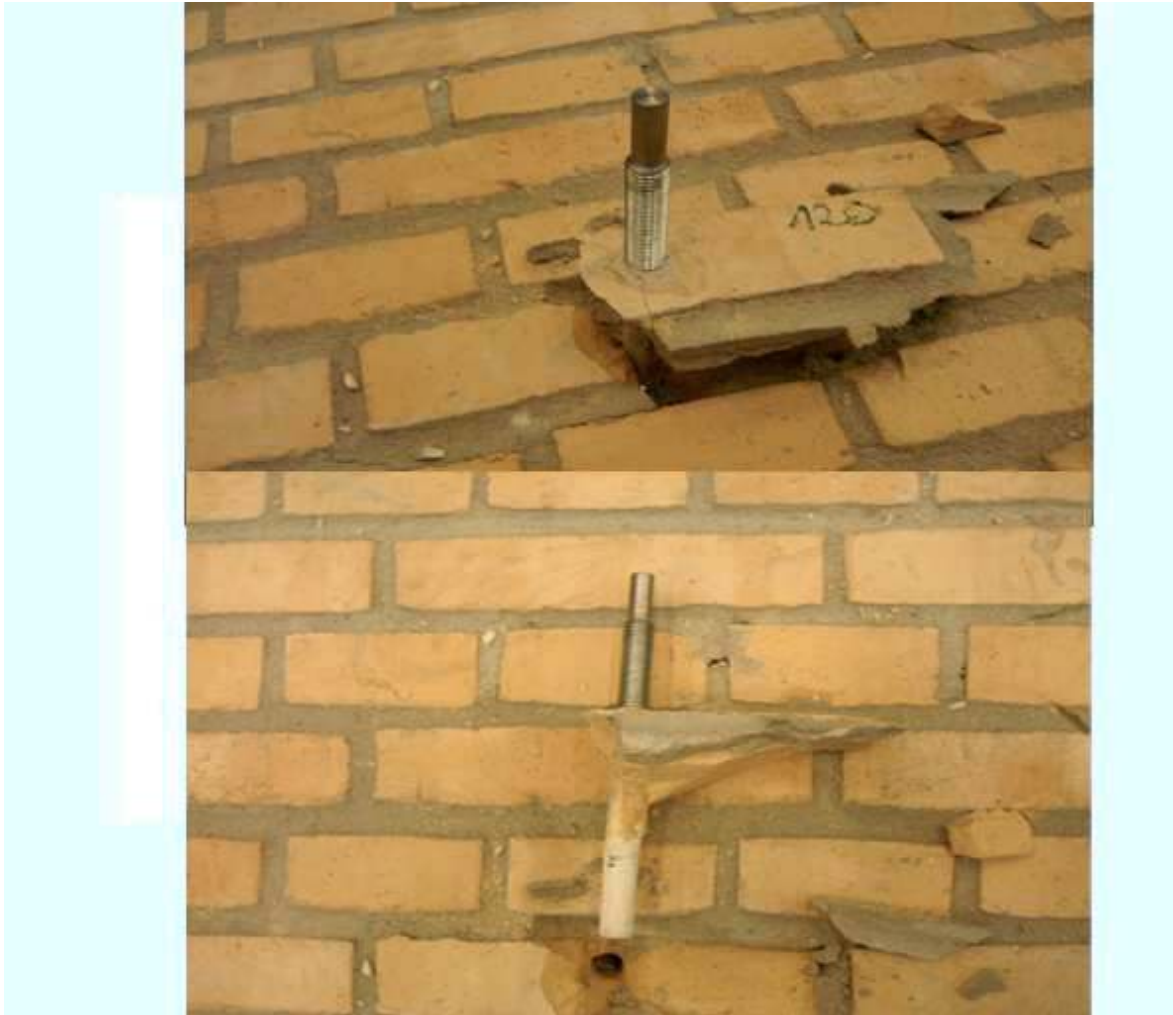
Figure A.33: The failure mode observed
