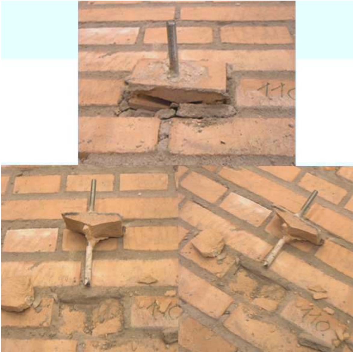
Figure A.55: The failure mode observed
