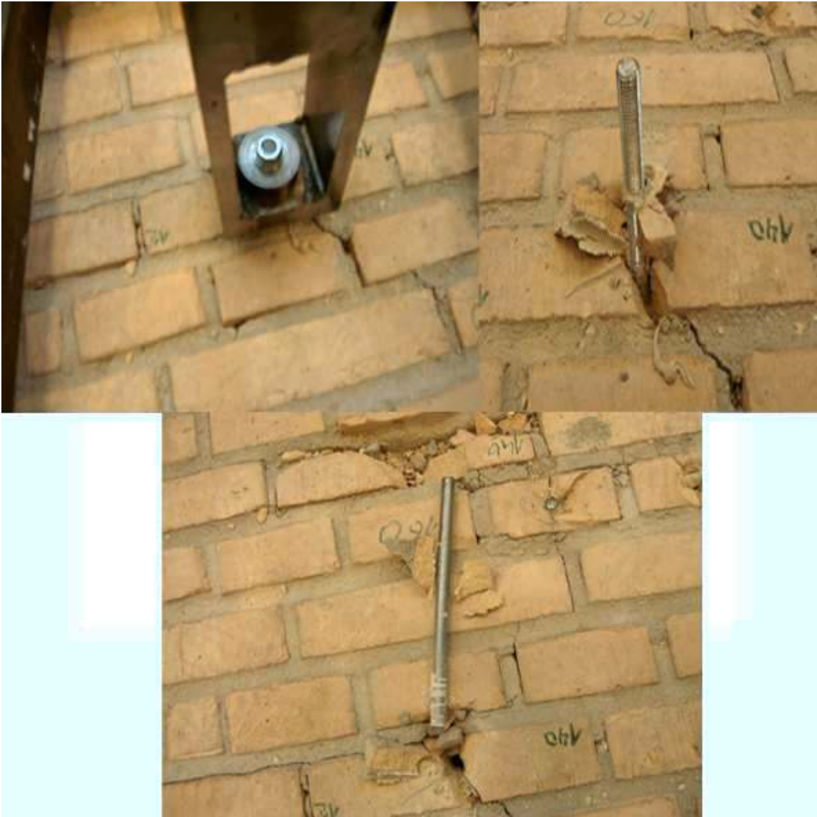
Figure A.27: The failure mode observed
