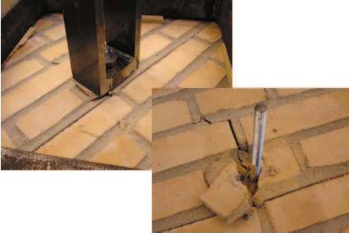
Figure A.41: The failure mode observed
