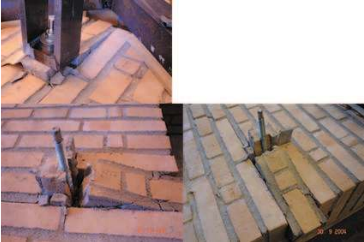
Figure A.137: The failure mode observed
