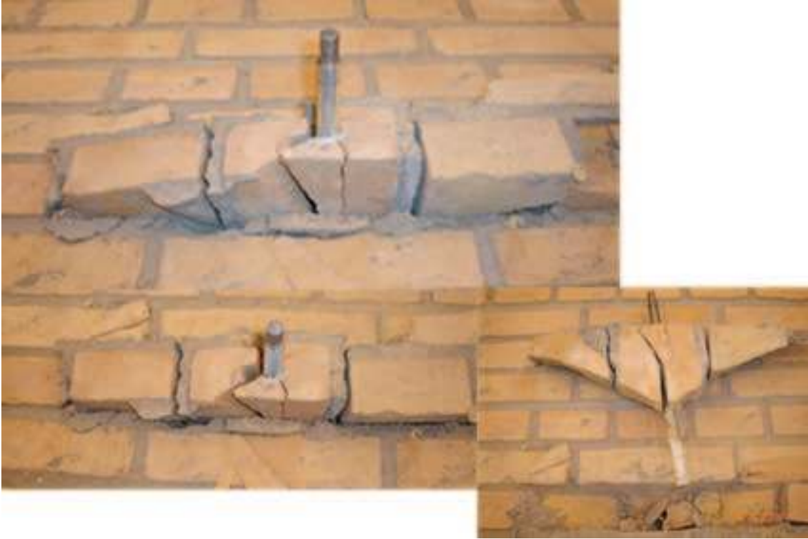
Figure A.49: The failure mode observed
