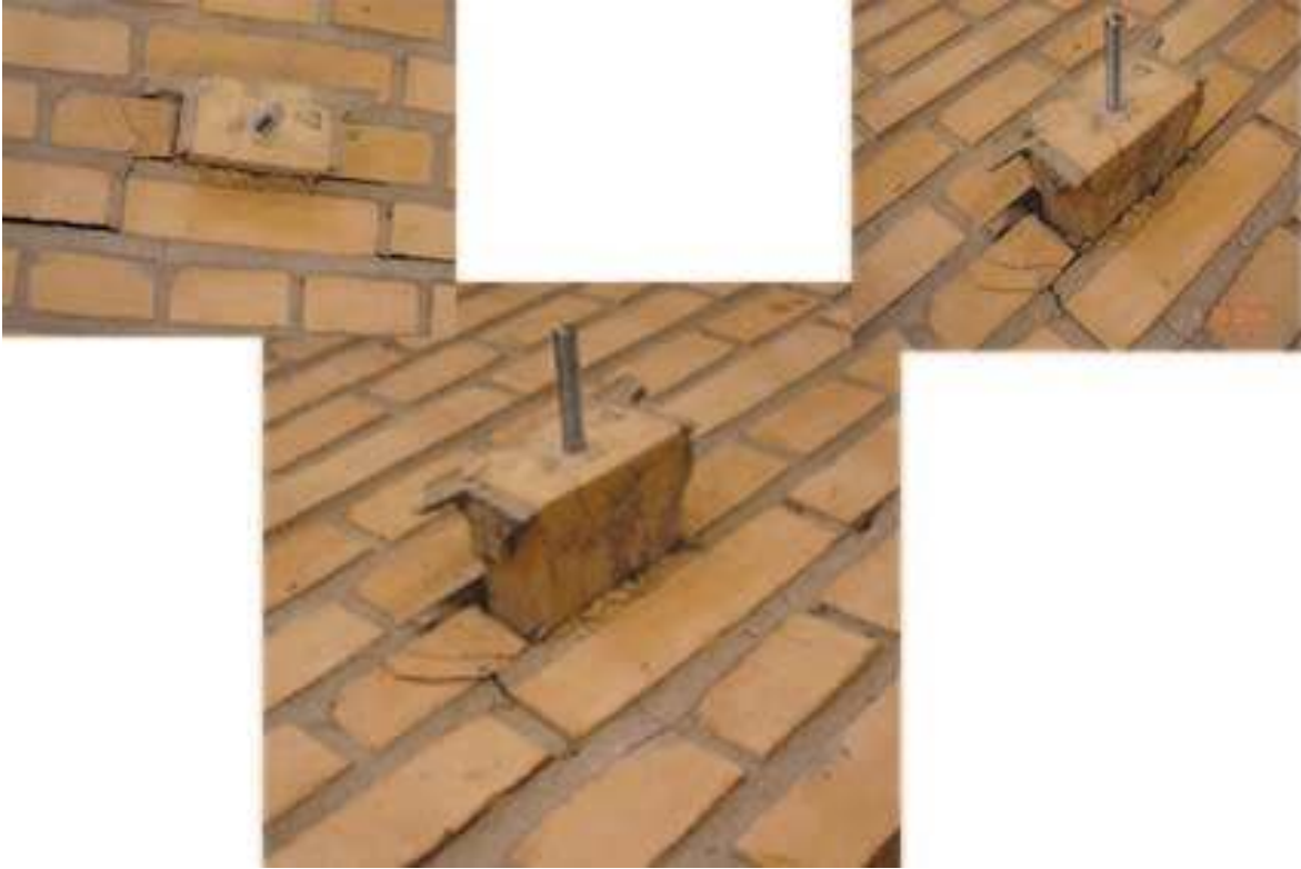
Figure A.143: The failure mode observed
