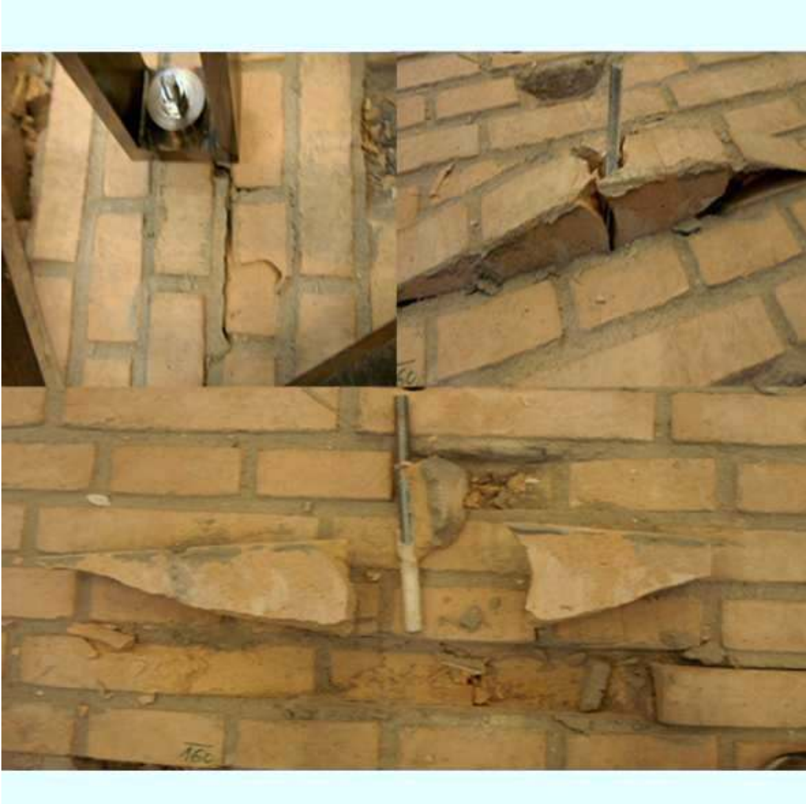
Figure A.29: The failure mode observed
