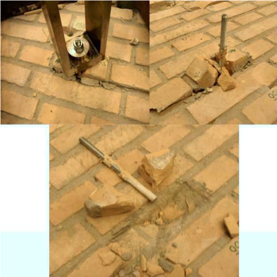
Figure A.73: The failure mode observed
