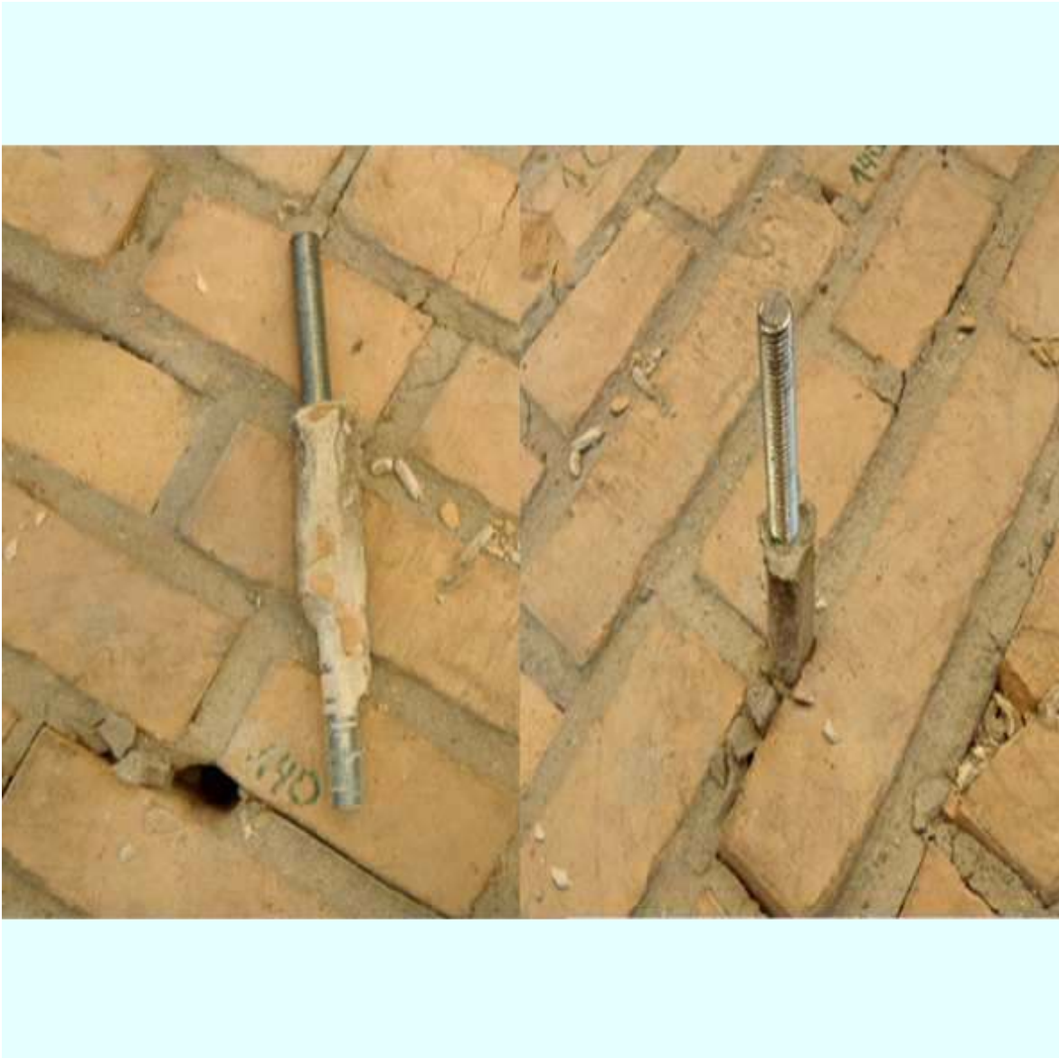
Figure A.97: The failure mode observed
