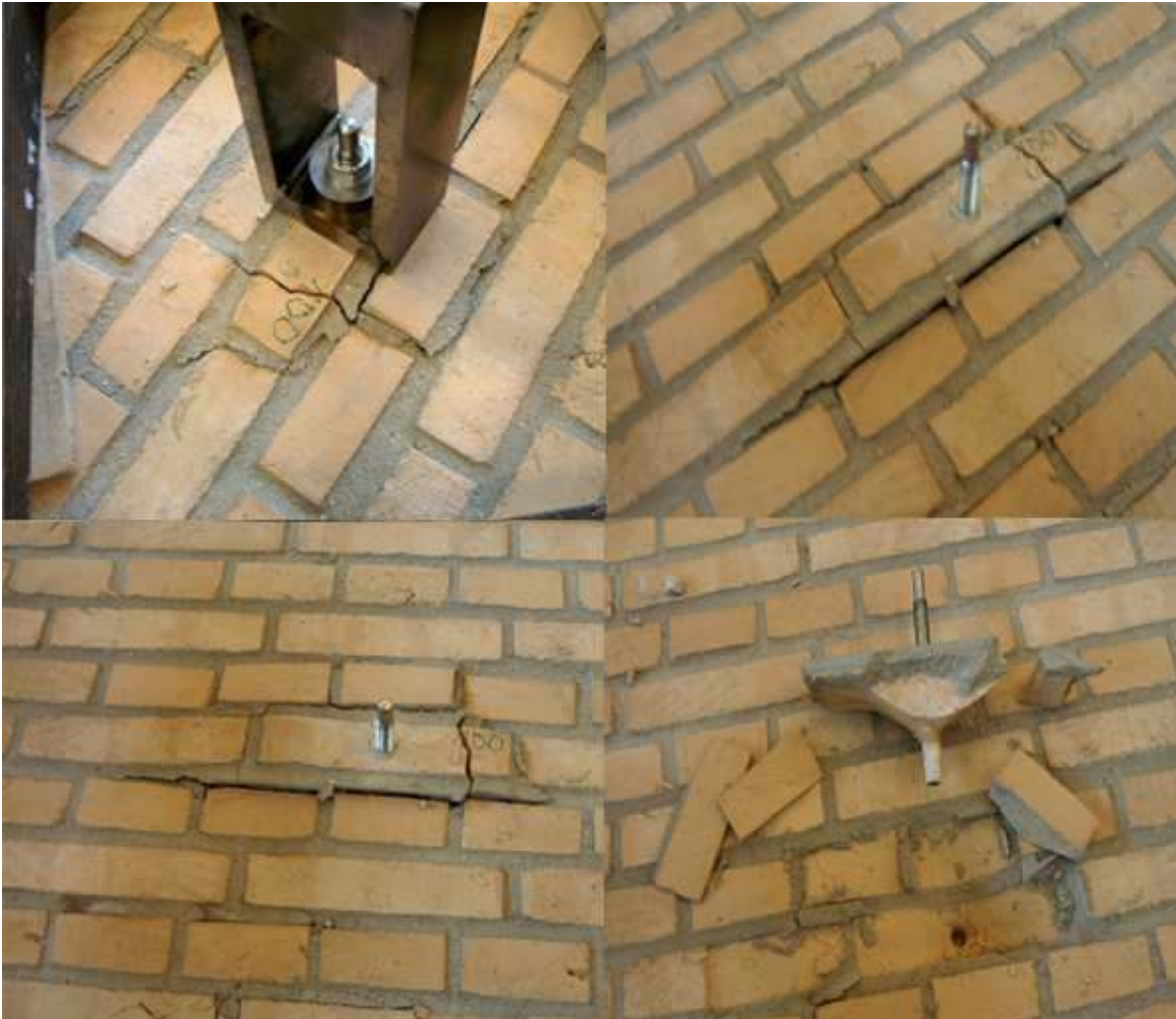
Figure A.31: The failure mode observed
