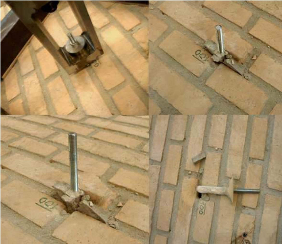
Figure A.85: The failure mode observed
