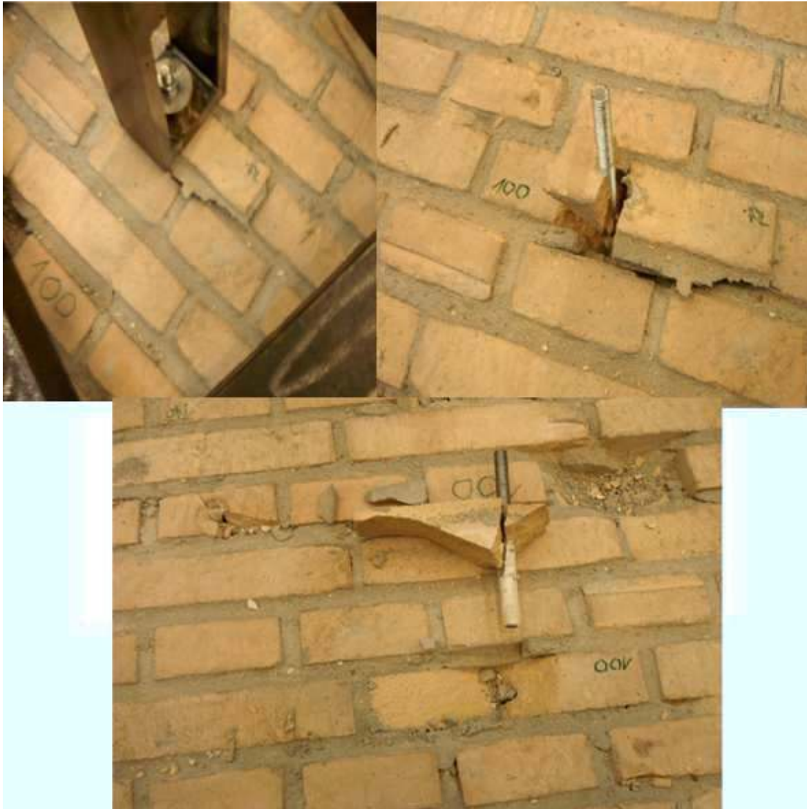
Figure A.23: The failure mode observed
