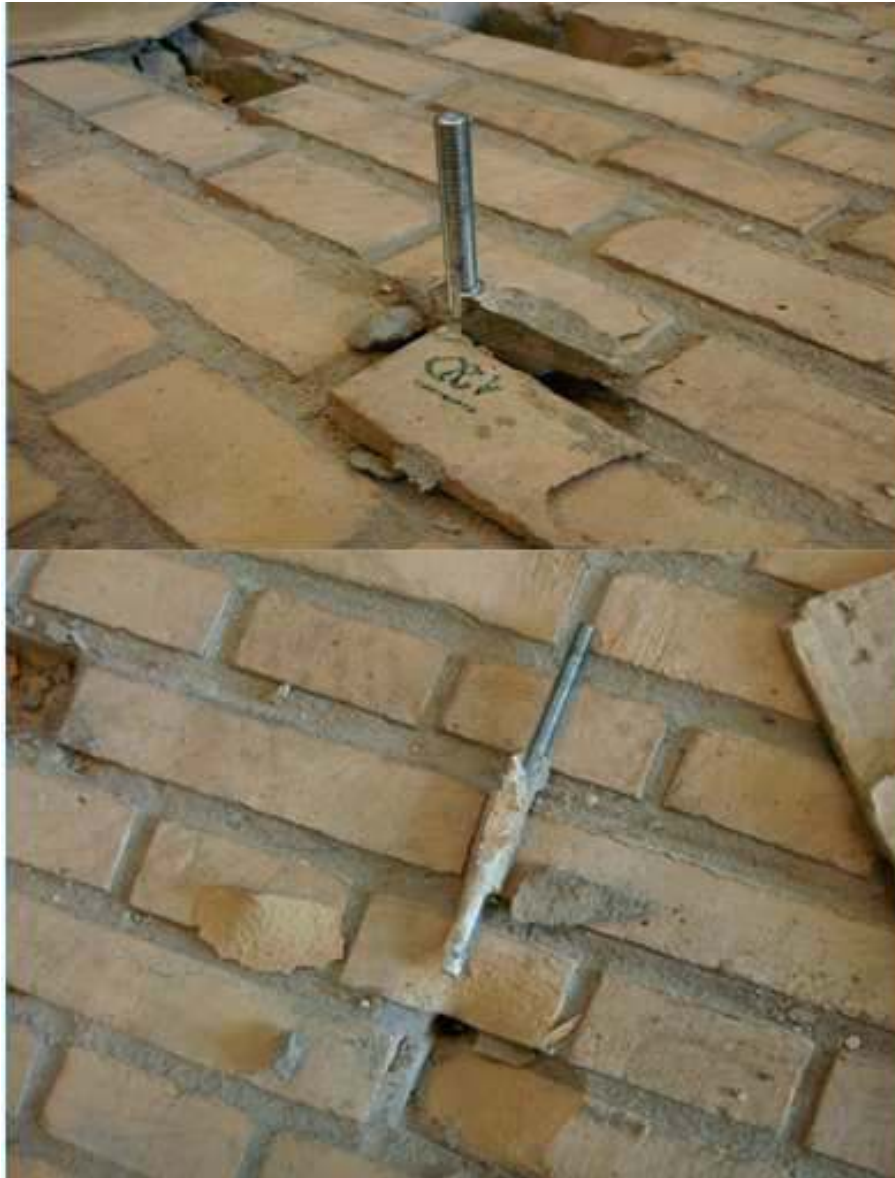
Figure A.87: The failure mode observed
