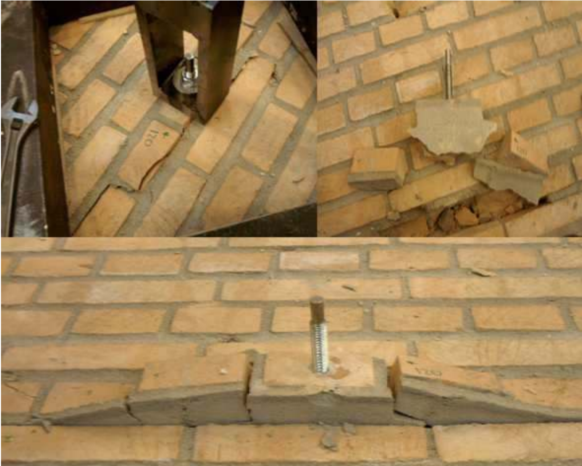
Figure A.79: The failure mode observed
