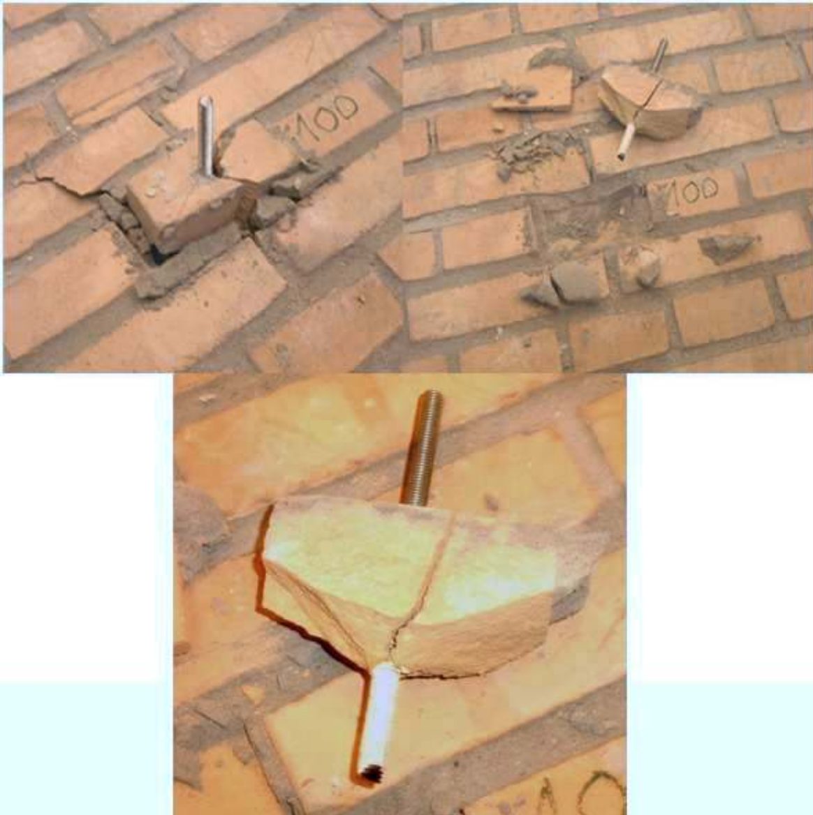
Figure A.53: The failure mode observed
