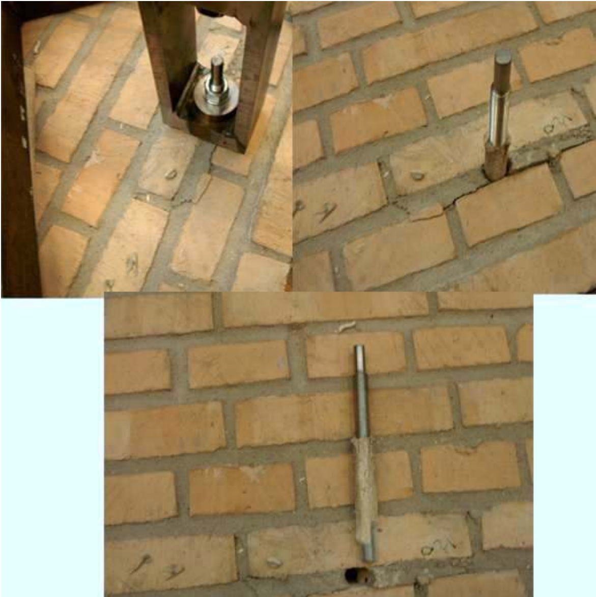
Figure A.103: The failure mode observed
