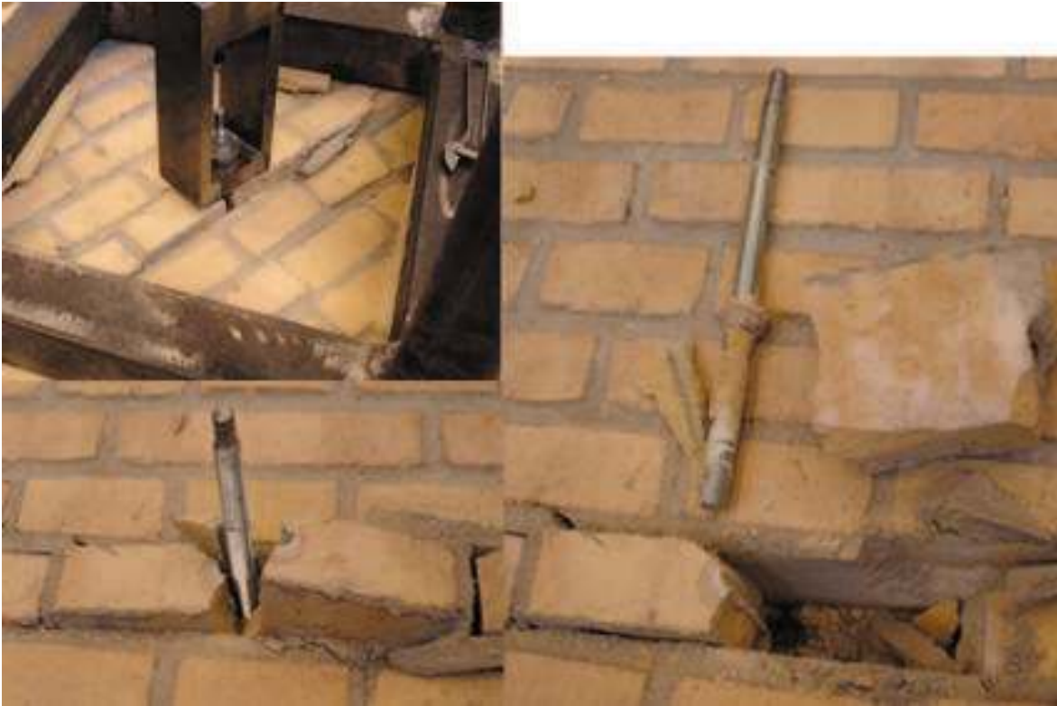
Figure A.11: The failure mode observed
