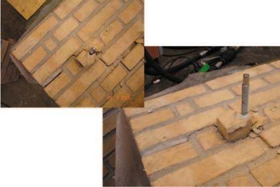
Figure A.123: The failure mode observed
