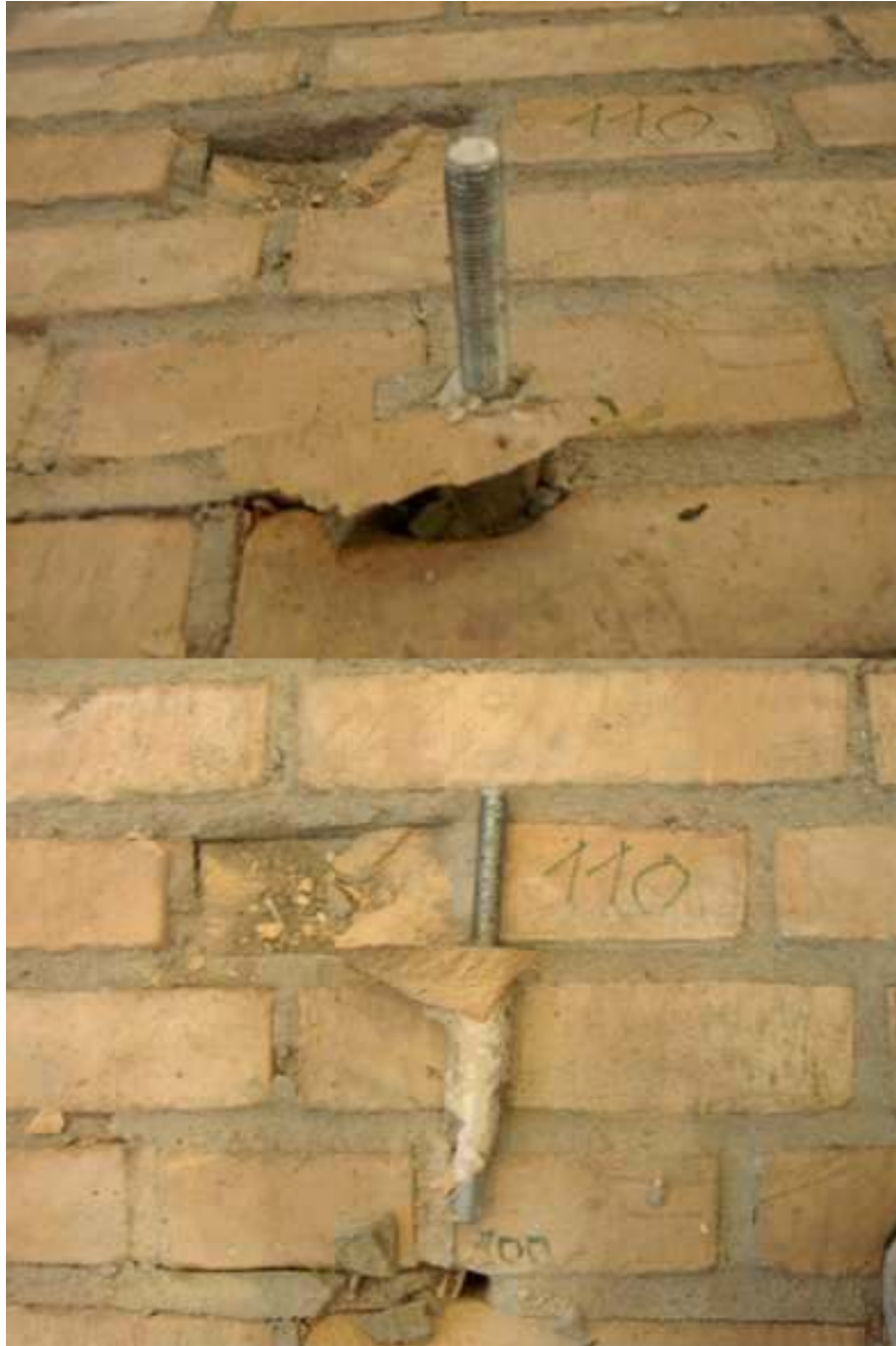
Figure A.93: The failure mode observed
