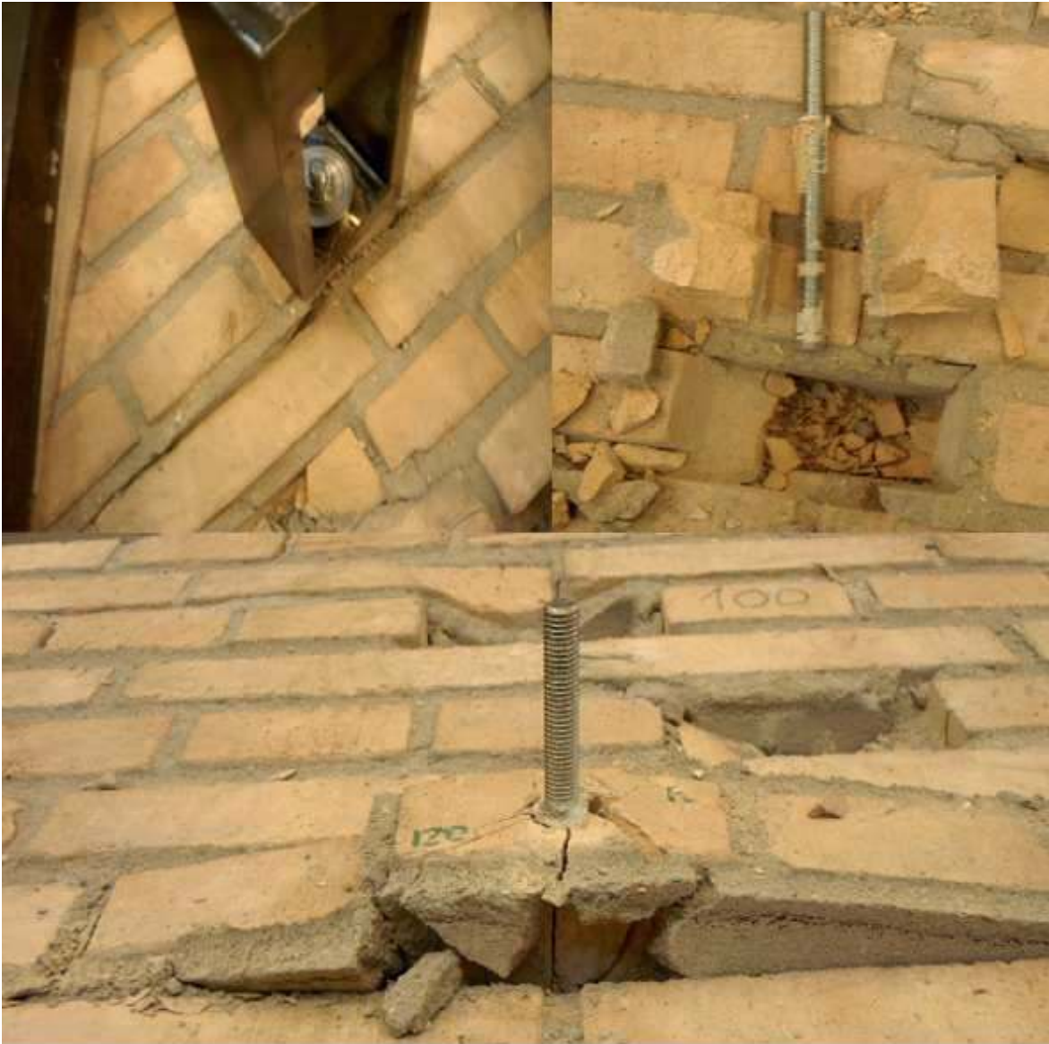
Figure A.71: The failure mode observed
