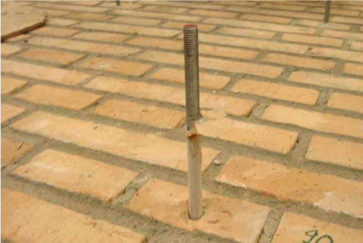
Figure A.51: The failure mode observed
