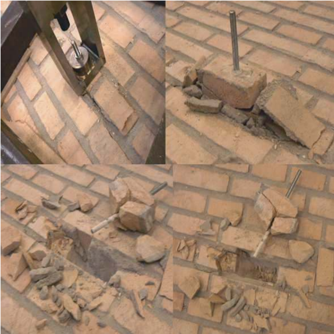
Figure A.67: The failure mode observed
