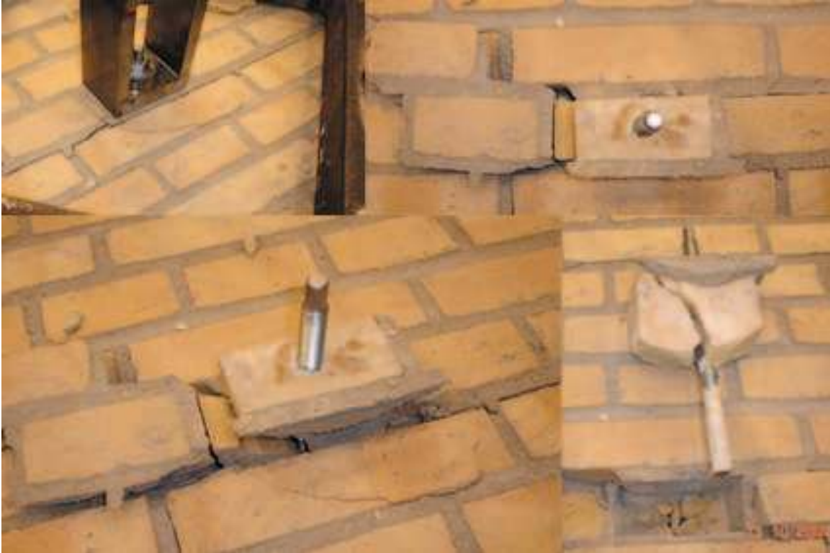
Figure A.47: The failure mode observed
