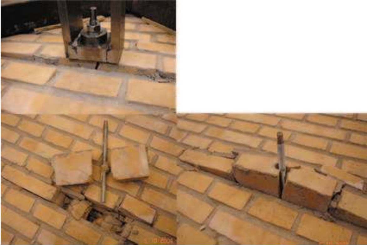
Figure A.13: The failure mode observed
