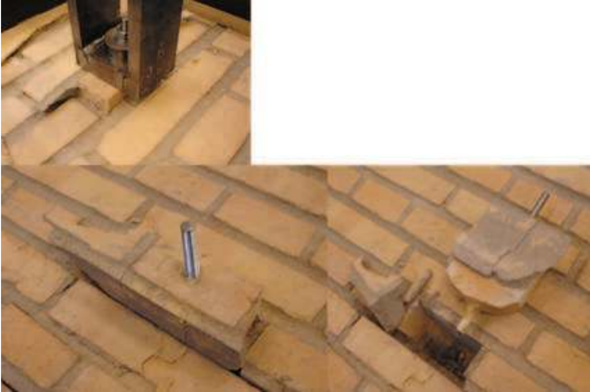
Figure A.39: The failure mode observed
