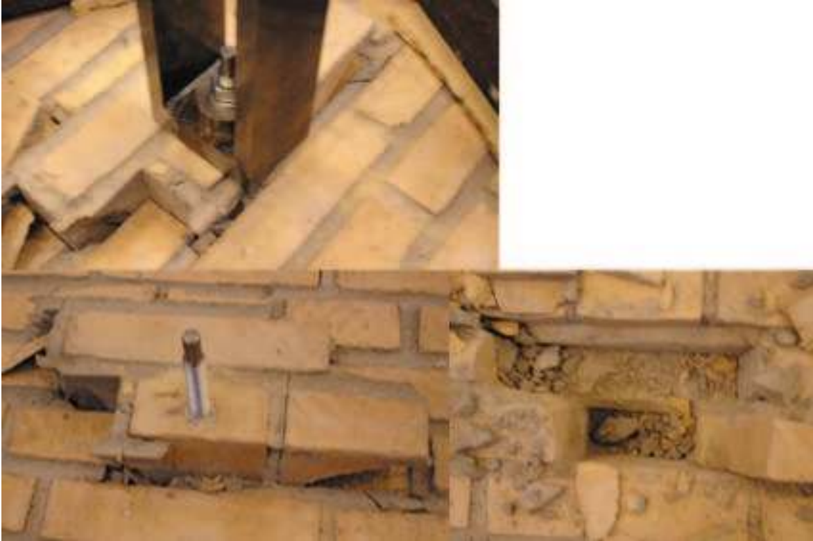
Figure A.45: The failure mode observed
