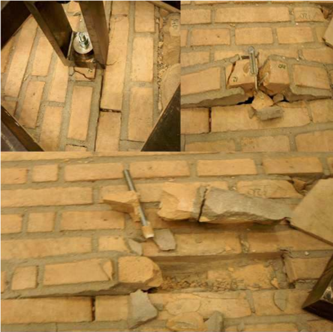
Figure A.69: The failure mode observed
