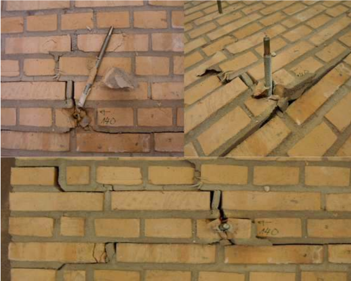
Figure A.81: The failure mode observed
