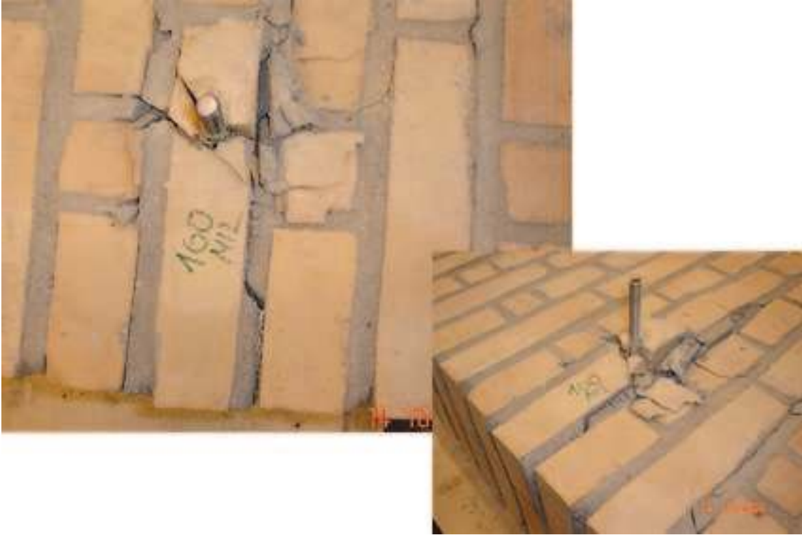
Figure A.129: The failure mode observed
