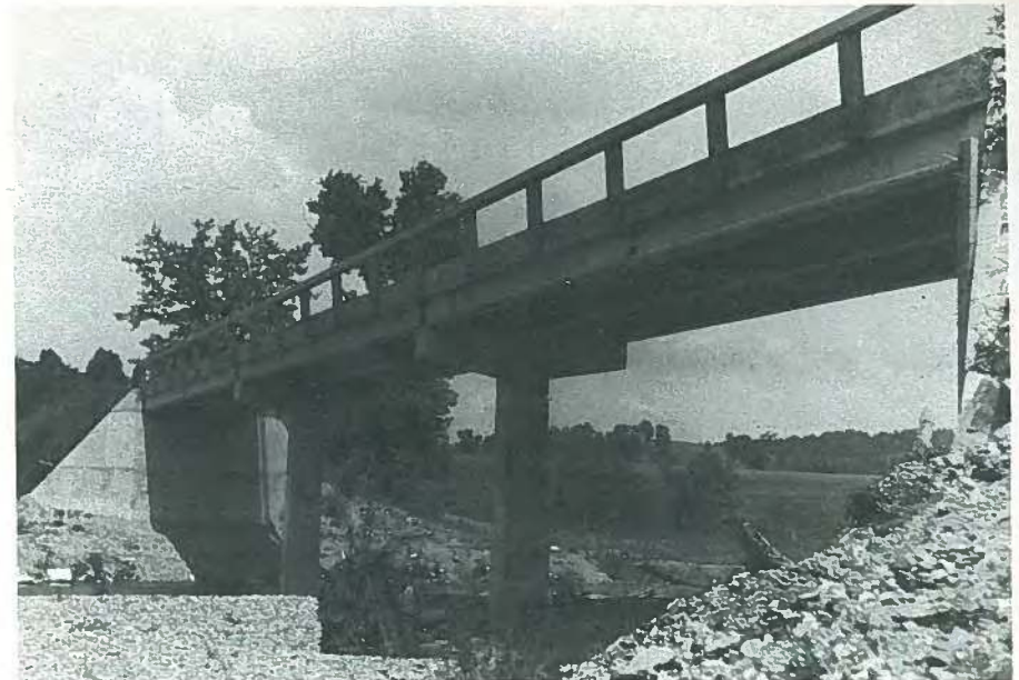
Fig. 18. Cheatham County Bridge of three 50-ft (15.3 m) spans made continuous by reinforcing in composite pour over supports. Pier caps are precast. Built in 1955.
