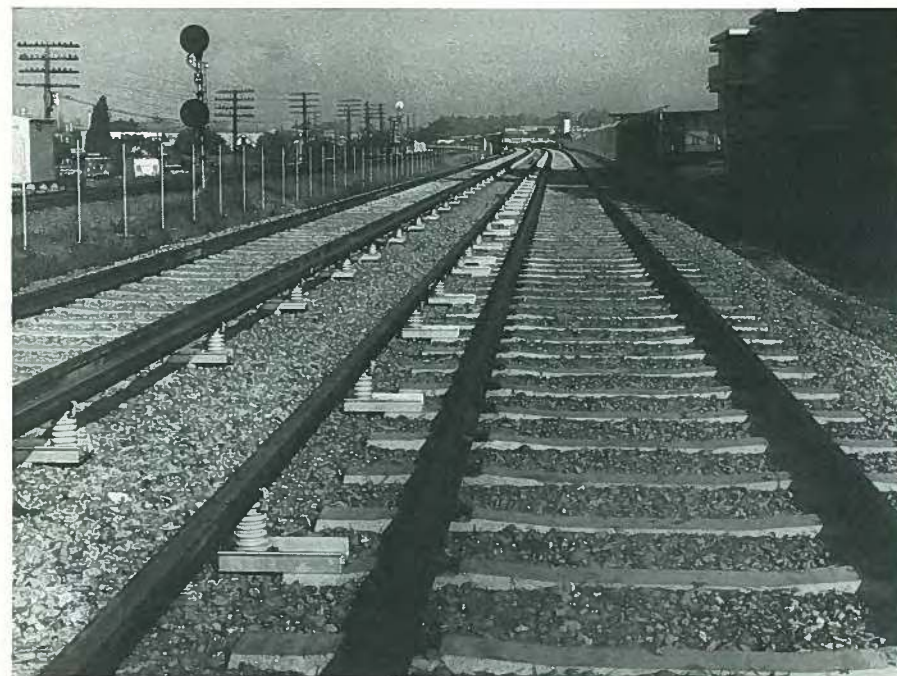
Fig. 53. Gerwick RT-2 type crossties as installed into Bart track system at Hayward, California.
