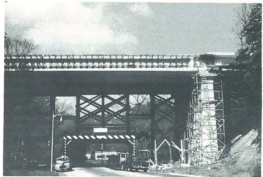
Fig. 1. The Walnut Lane Bridge under construction in 1950. Photograph shows brackets in place for formwork for sidewalk at south fascia girder.
