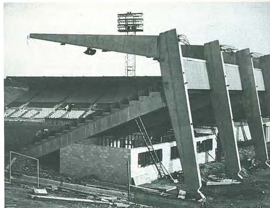
Fig. 68. Cheney Stadium in Tacoma, completed in 3½ months, did much to publicize the usefulness of prestressed concrete.
