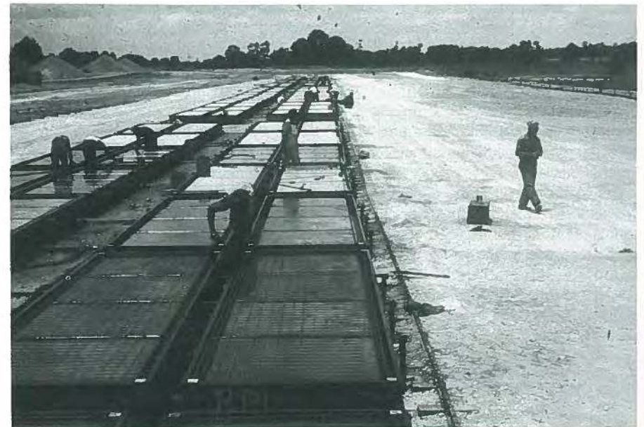
Fig. 26. Precast concrete installation at the U.S. Marine Corps Supply Depot in Albany, Georgia, 1952. One hundred and forty concrete molds permitted a daily production of 140 thin shell ribbed roof panels required for the 10 warehouses shown in the section above (Fig. 25).
