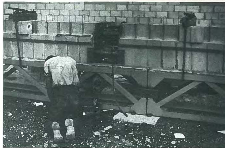
Fig. 10. Tensioning two 16x24-in. (406 x 610 mm) block building beams by jacking them apart.
