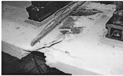
a) Concrete Crushing
