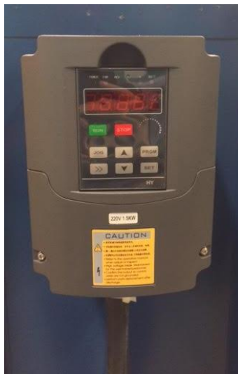
Figure 3.7. Huanyang variable frequency drive operator interface.
