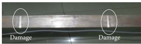
FIGURE 3: Damages in experimental beam.
