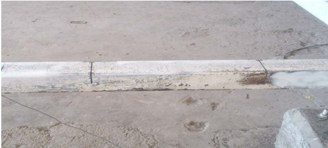
Figure 22 - Second damage scenario
