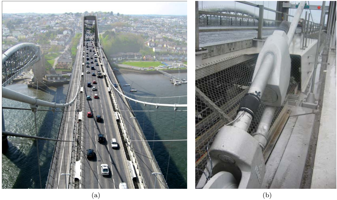
Figure 9: Shear boxes shown behind the hanger sockets (left) and additional stay connection at deck level with strain-gauges (right)
