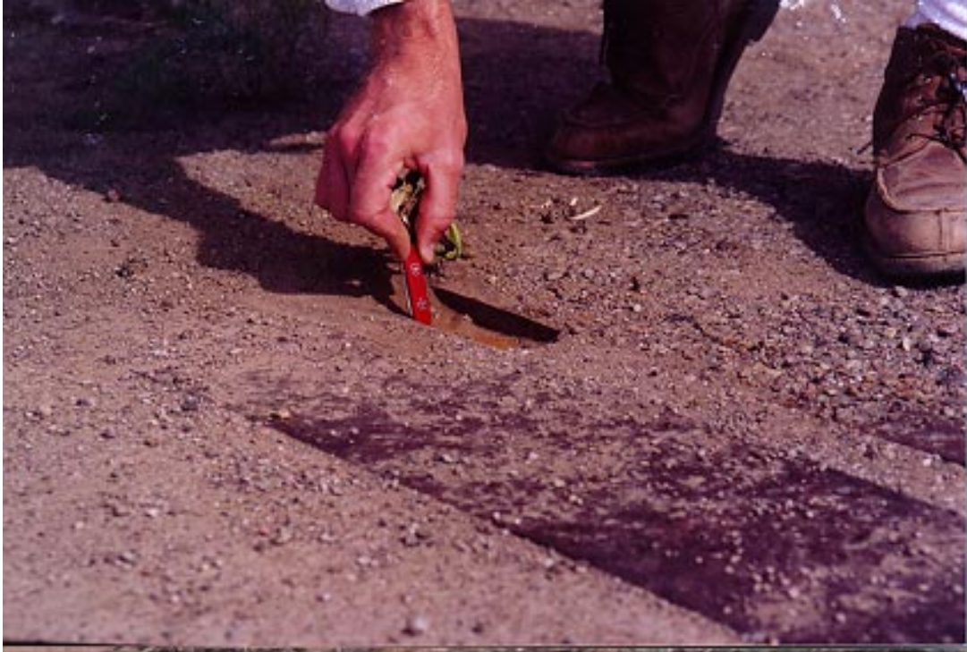
Figure 14. Debris in expansion joint at the north end of the bridge.
