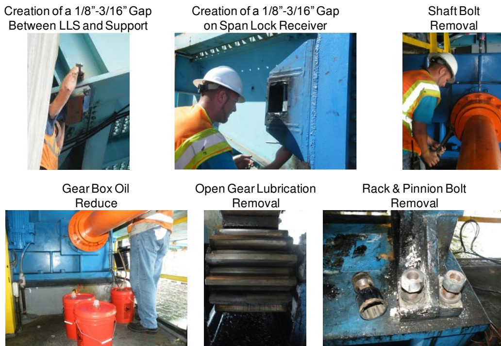
Figure 19: Damage tests on Sunrise Boulevard Bridge
