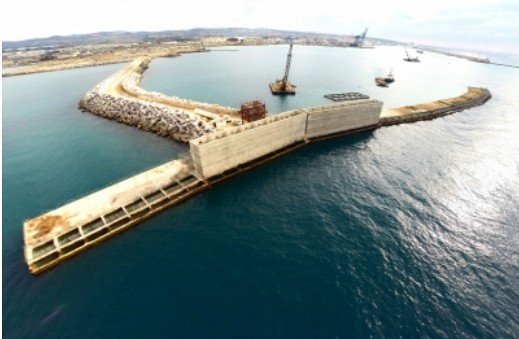
Figure 2.2: The new breakwater of the port of Civitavecchia during construction, showing the individual caissons. [21]
