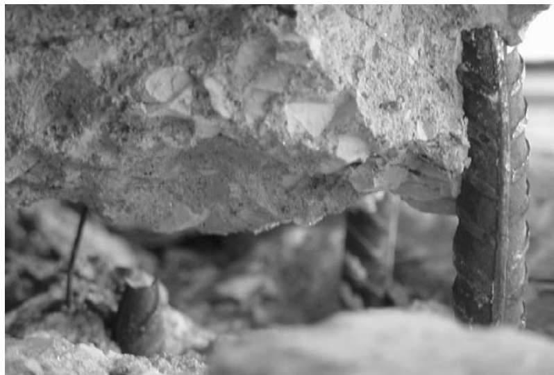
Fig. 2 Failure of steel bars of the column and slipping of steel bars of the added jacketing
